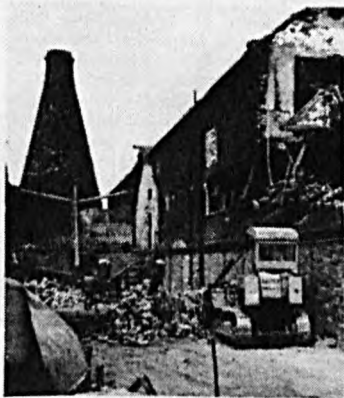
Fig. 5—Last of two remaining ovens, polishing shop, now rubble, sorting and stock warehouses, demo' men moving in.
