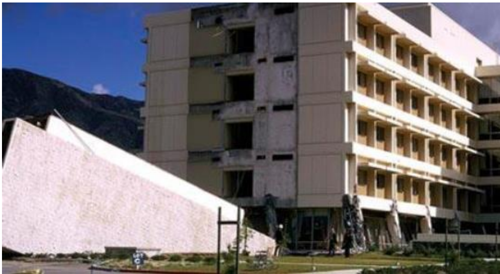
Figure 2.3 Olive view hospital pounding- the stairway collapsed sometime after the earthquake (Mahin and Bertero, 1976)
