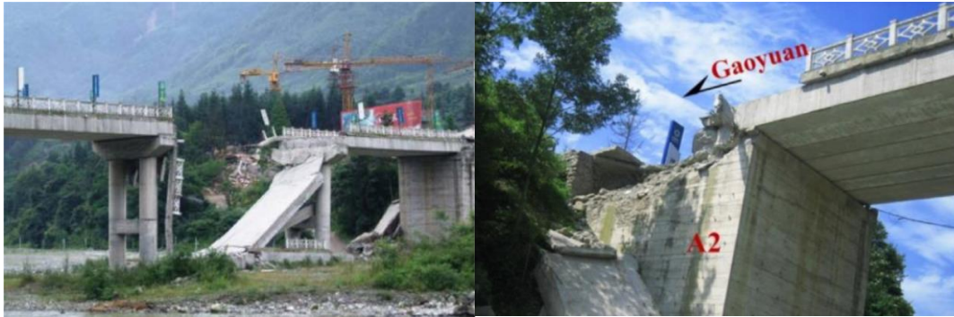
Figure 2.15 Gaoyuan Bridge pounding failure at expansion joints (Lin et al., 2010) as well as pounding of deck against abutments in Wenchuan earthquake (Hu et al., 2019)
