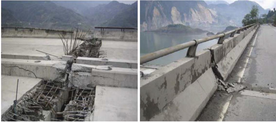
Figure 2.4 Earthquake induced pounding between bridge decks (Miari et al., 2019)
