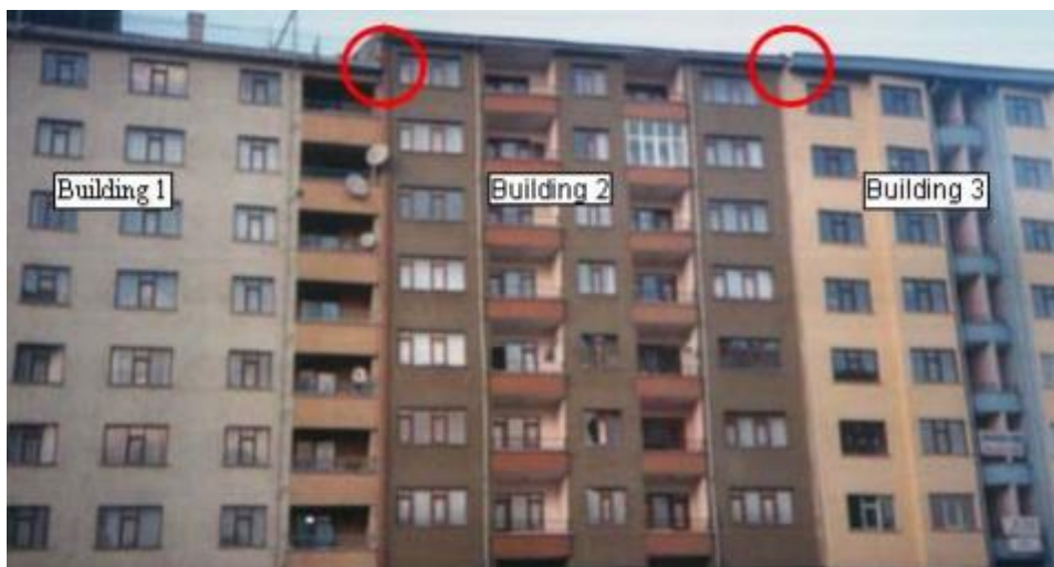
Figure 2.1 Adjacent buildings in Eskisehir city with insufficient gap as shown with red circle (Dogan and Gunaydin, 2009)
