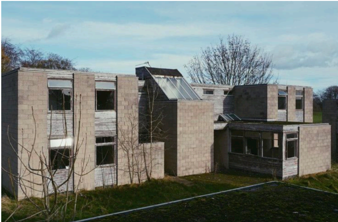
Figure 1.1: The student accommodation block at Wentworth Woodhouse campus of Sheffield Polytechnic, now derelict
