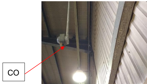
Figure 3.4 Ceiling level CO monitor in the Heaton railway depot
