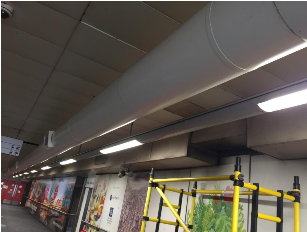
Figure 7.1 New ventilation system at the Manchester Victoria station in the overbridge section
