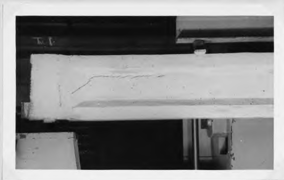
Plate 16 Cracking at the junction of the web and the upper flange
