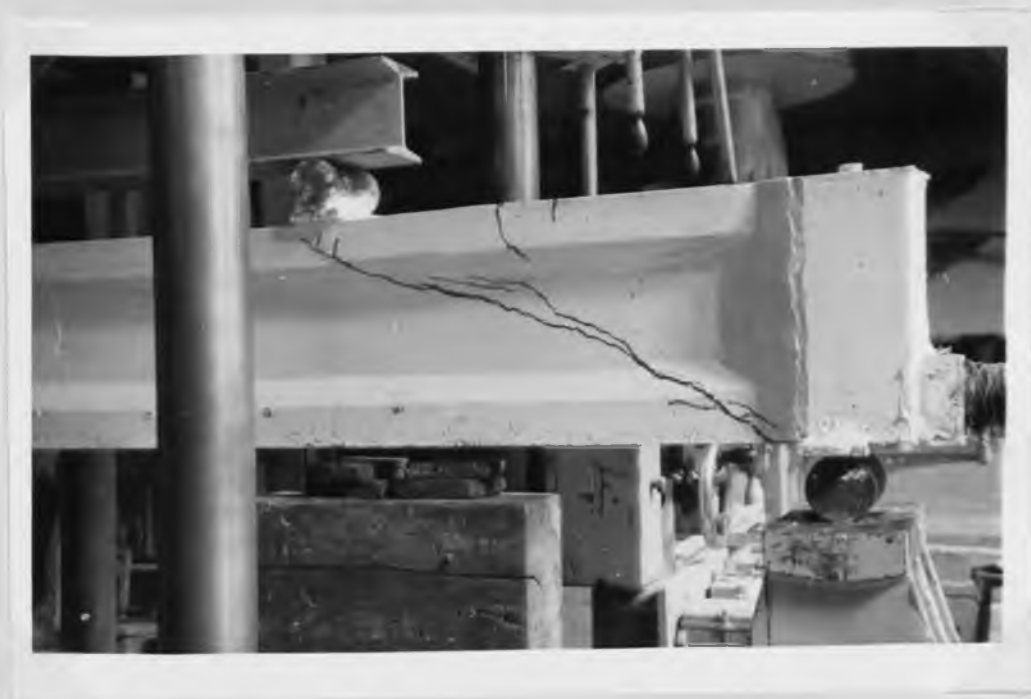
Plate 12 Vertical cracking in the upper flange following diagonal cracking
