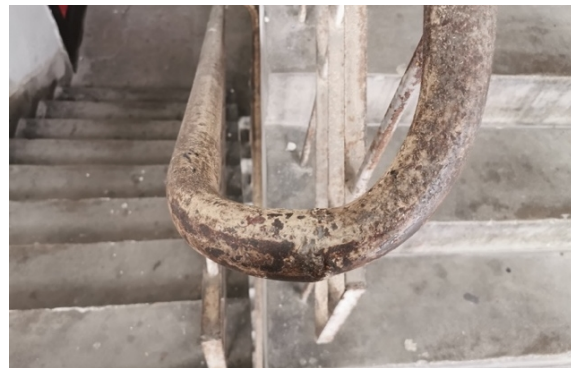
f. The rusty handrail
