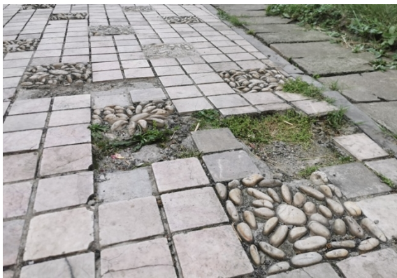
Uneven floor in roof garden
