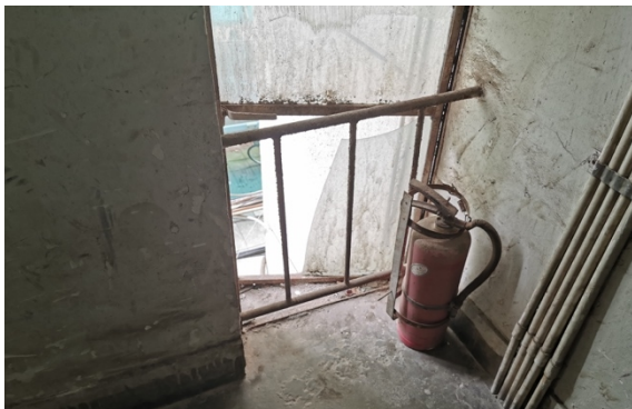
e. The broken glass on stair platform
