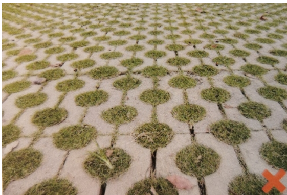
The gap between brick is large, not suitable for pavements.
