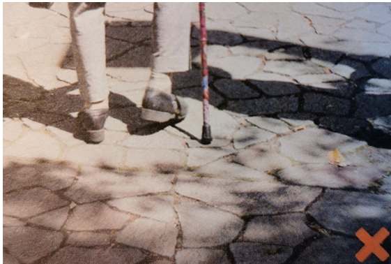
Fragmented, uneven ground surfaces are not suitable for pavements.
