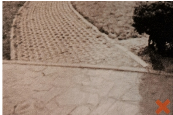
Older people may be trip up due to gap protrusions in a pavement junction with different materials.
