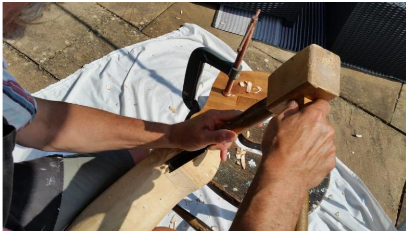
(Fig. 10.19 mortise chiselling and gouging of the joint ends, author's own image)
