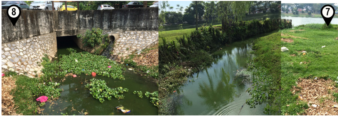
Figure 6.35 The outlet that allows excess water to flow from the lake to the river faces issues with wild aquatic plants and trapped rubbish
