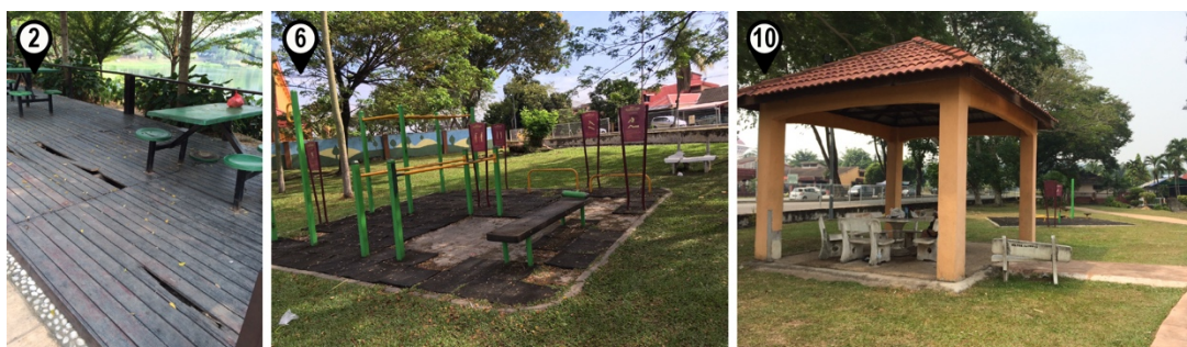
Figure 6.49 The broken and damaged facilities and equipment in the park are perceived to be 'dangerous' to the users and hinderances to the utilisation of these spaces
