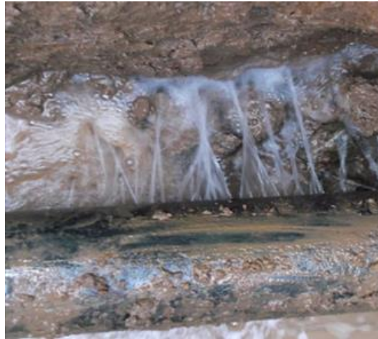
Figure 1-4 Erosion and void formation around a breached pipe (Water matters UK.2013)
