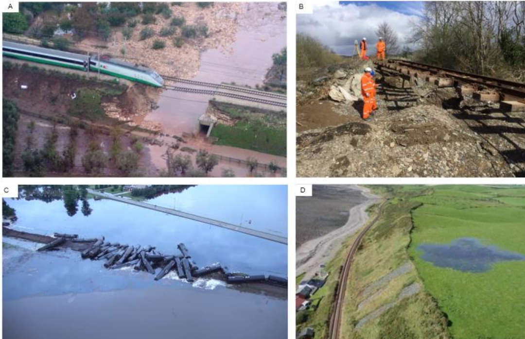
Figure 6: Illustrations of rail slopes subjected to flooding: a) embankment failure following offset head flooding in Acquivavia, Italy (October 2005); b) Embankment failure in Conwy, UK, following overtopping flood (March 2019); c) failure of embankment following train loading during basal flooding in Ohio, USA (June 2018); d) floodwater development above slope, causing infiltration in UK (a) reproduced from Polemio and Lollino (2011); b) and d) courtesy of Network Rail; c) courtesy of Sioux County Sherriff.
