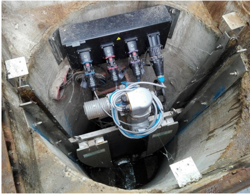
Figure 2.6: CENTAUR flow control device installed in the Coimbra combined sewer network (Portugal).
