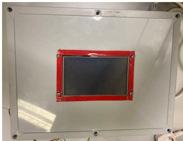
Figure 6.24: Touchscreen mounted on electrical enclosure lid.
