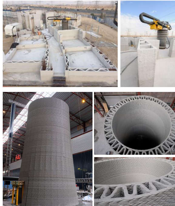
Figure 6.1 Some applications of the additively manufactured concrete. On the top: a robotic printer constructing a 640m 2 and 9.5 m high building (image from Apis Cor). Bottom: additive manufacturing of 10 m base of wind turbines (image from COBOD).
