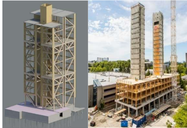
Figure 2-9: Timber-concrete hybrid building: timber frame with a concrete slab(left)(Malo et al., 2016), timber frame with concrete core (right) ( https://www.naturallywood.com/resource/introduction-to-brock-commons-tallwood-house-ubc-tall-wood-building/ )
