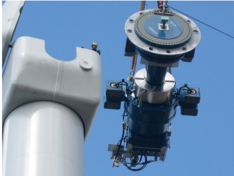
Figure 1.6: A gearbox, rotor shaft and brake assembly being installed in a wind turbine nacelle [24].
