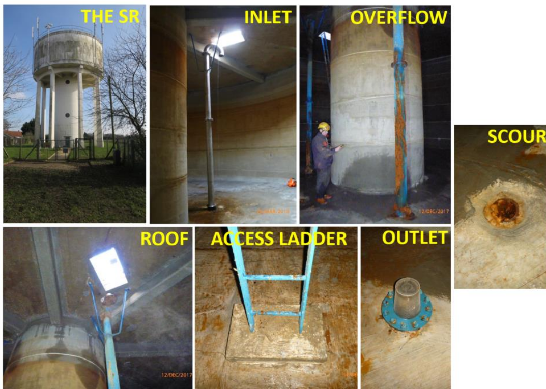
Figure 5.3 – Schematic of A1 SR and collection of photos displaying the external and internal details of the SR.
