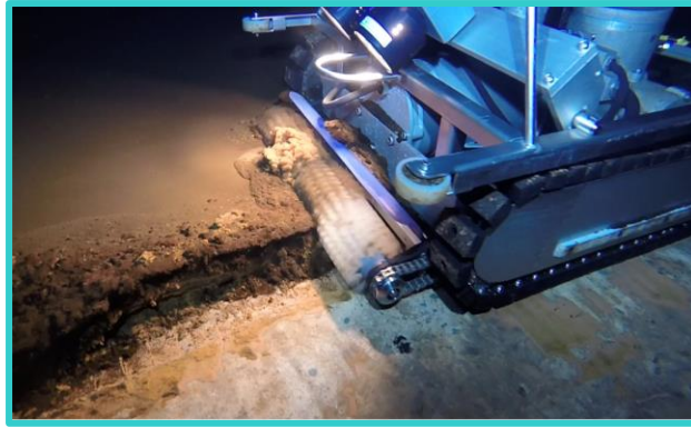
Figure 2.14 – A remotely operated vehicle removing accumulated material in a service reservoir. Image source: Panton McLeod.
