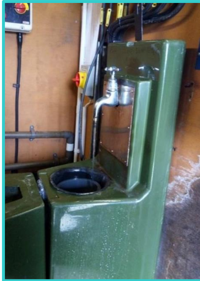
Figure 2.5 – An example of a regulatory service reservoir outlet sample tap.
