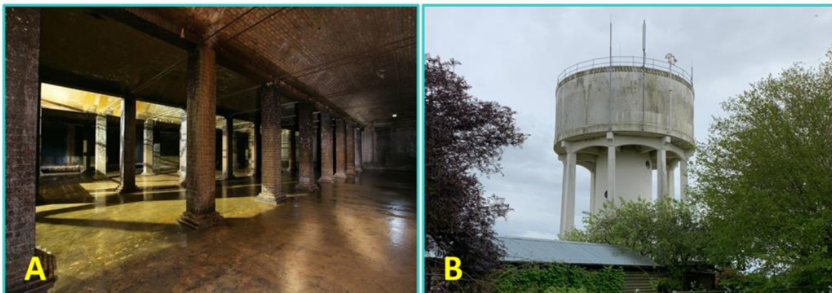
Figure 2.2 – An example of an underground service reservoir (A) and an overground water tower (B).
