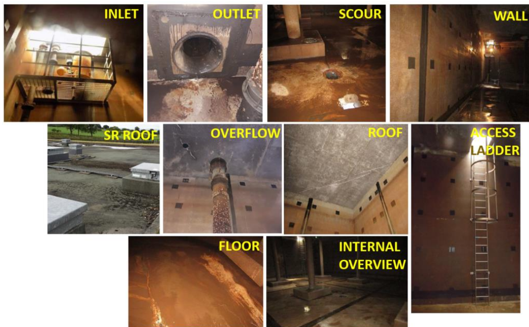
Figure 5.15 – A schematic of C3 SR A collection of photos displaying the external and internal details of the SR.
