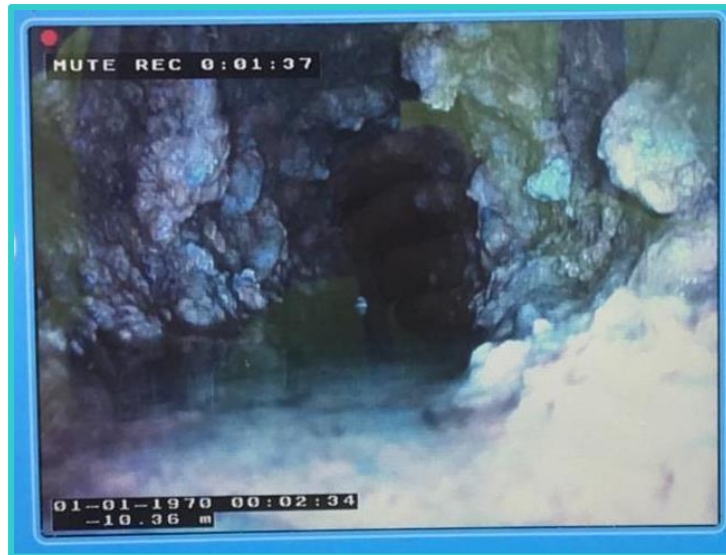
Figure 2.10 – A video still image of corroded scale on the inside of a pipe, which is visibly restricting its hydraulic capacity. Image source: Severn Trent Water.
