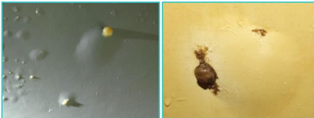
Figure 2.4 – An example of blistering and biofilm growth on glass reinforced plastic service reservoir walls. Image source: UKWIR (left) and Northumbrian Water (right).
