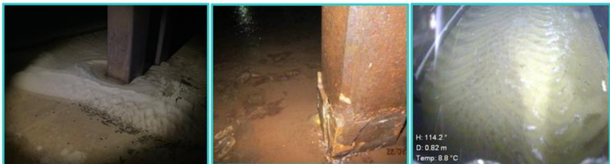
Figure 2.7 – Examples of accumulated material from three different service reservoirs. Image source (from left to right): Severn Trent Water, Northumbrian Water, and Panton McLeod.
