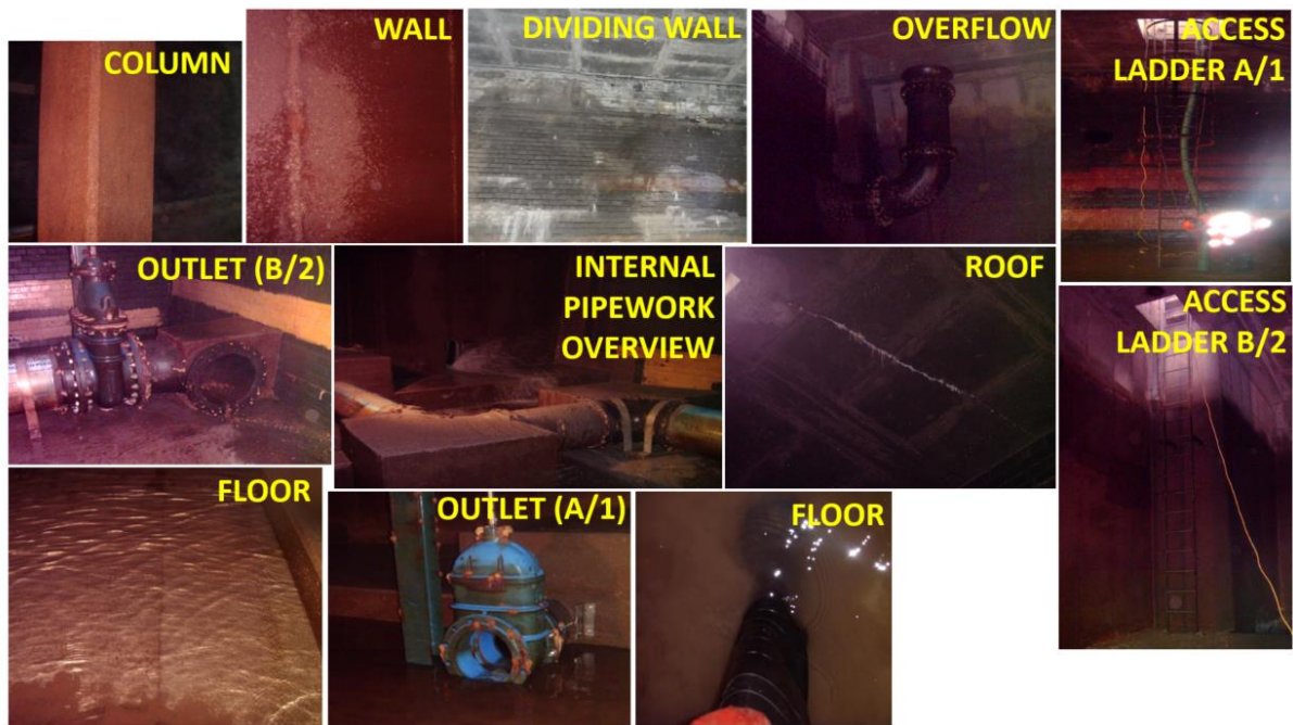
Figure 5.24 – A schematic of D4 SR and a collection of photos displaying the internal details of the SR.
