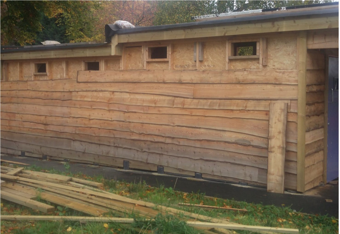
Figure 6.25. A shed, workshop and bin store with a green roof was designed and built by a small working group of residents.
