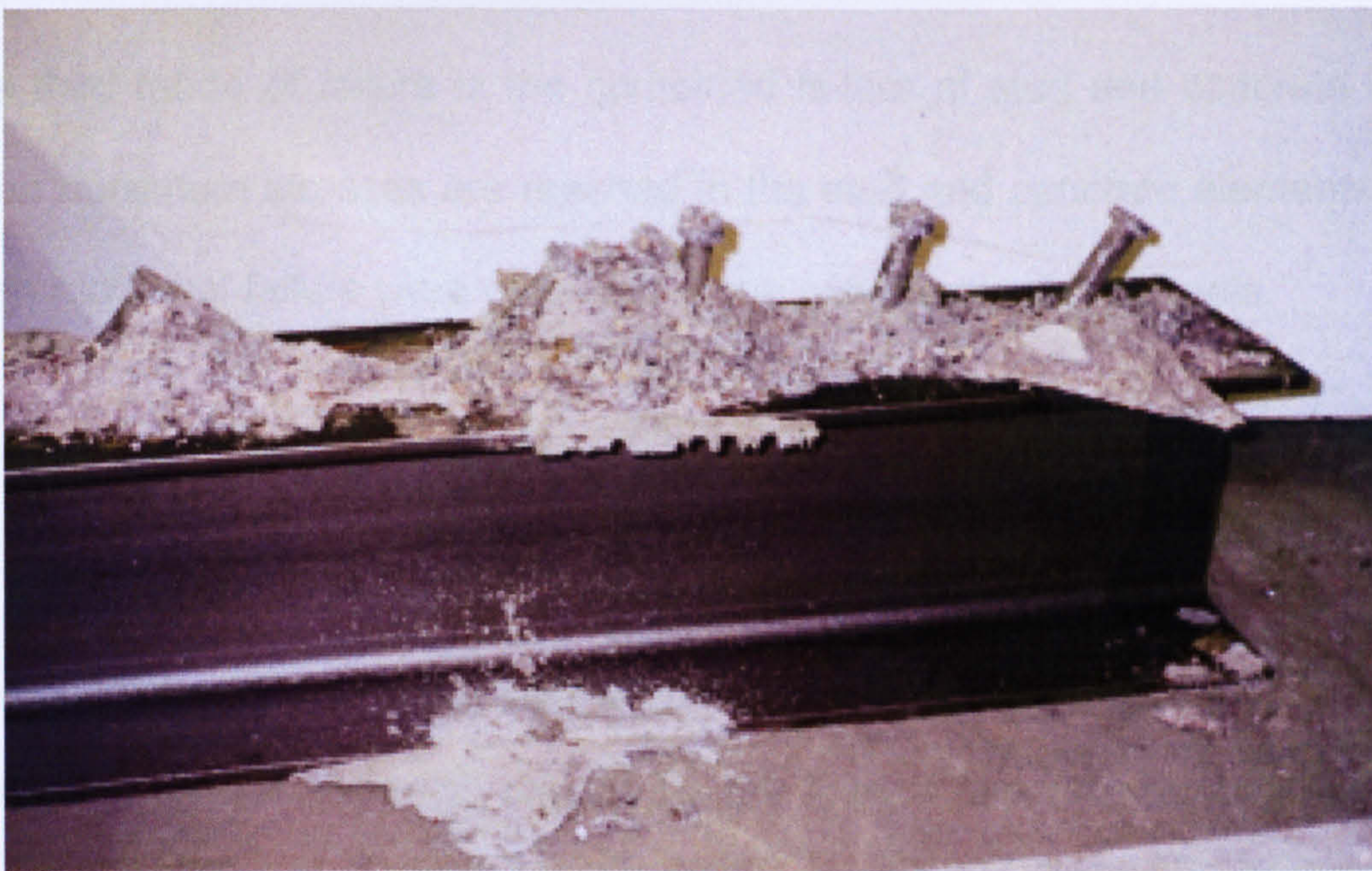
Figure 4.1: Crushing of concrete/conical failure
