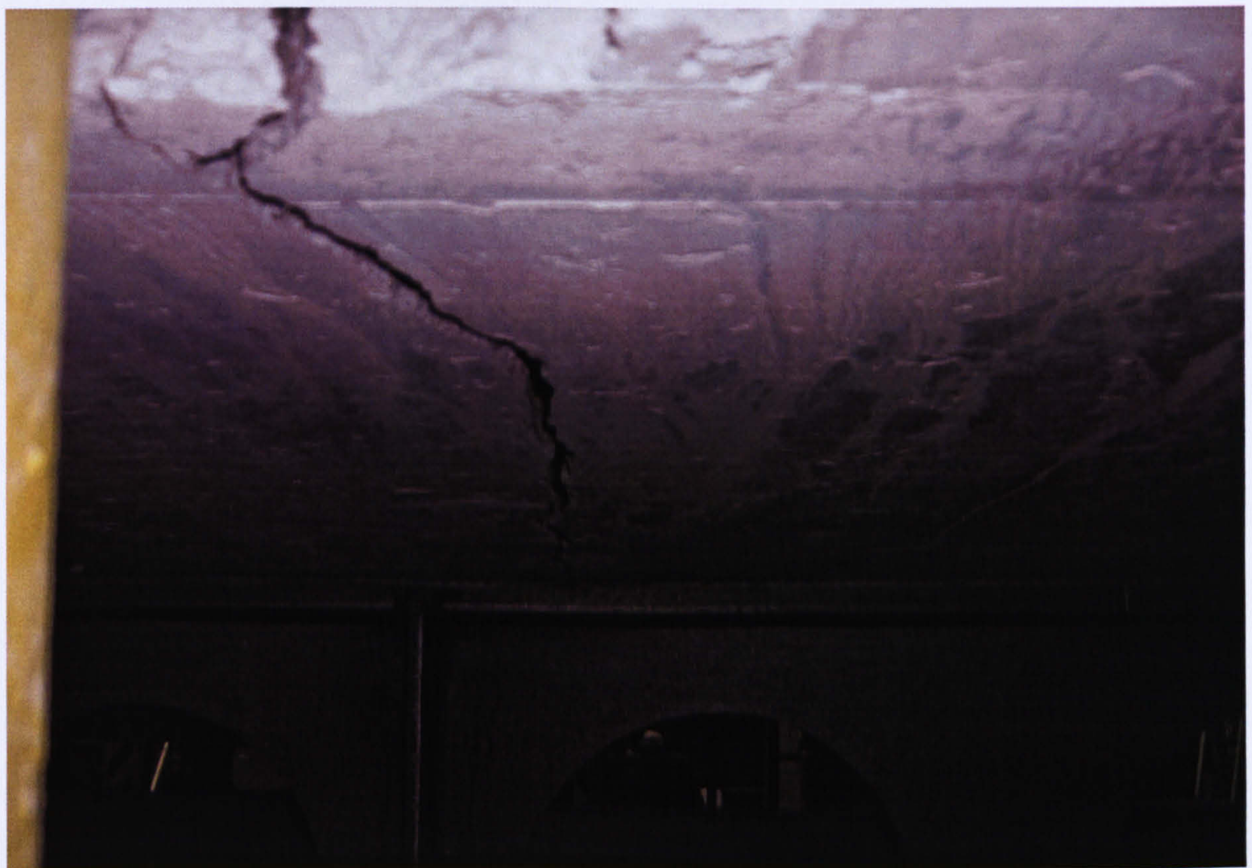
Figure 4.42: Excessive cracking on underside slab of CB-5 (East)
