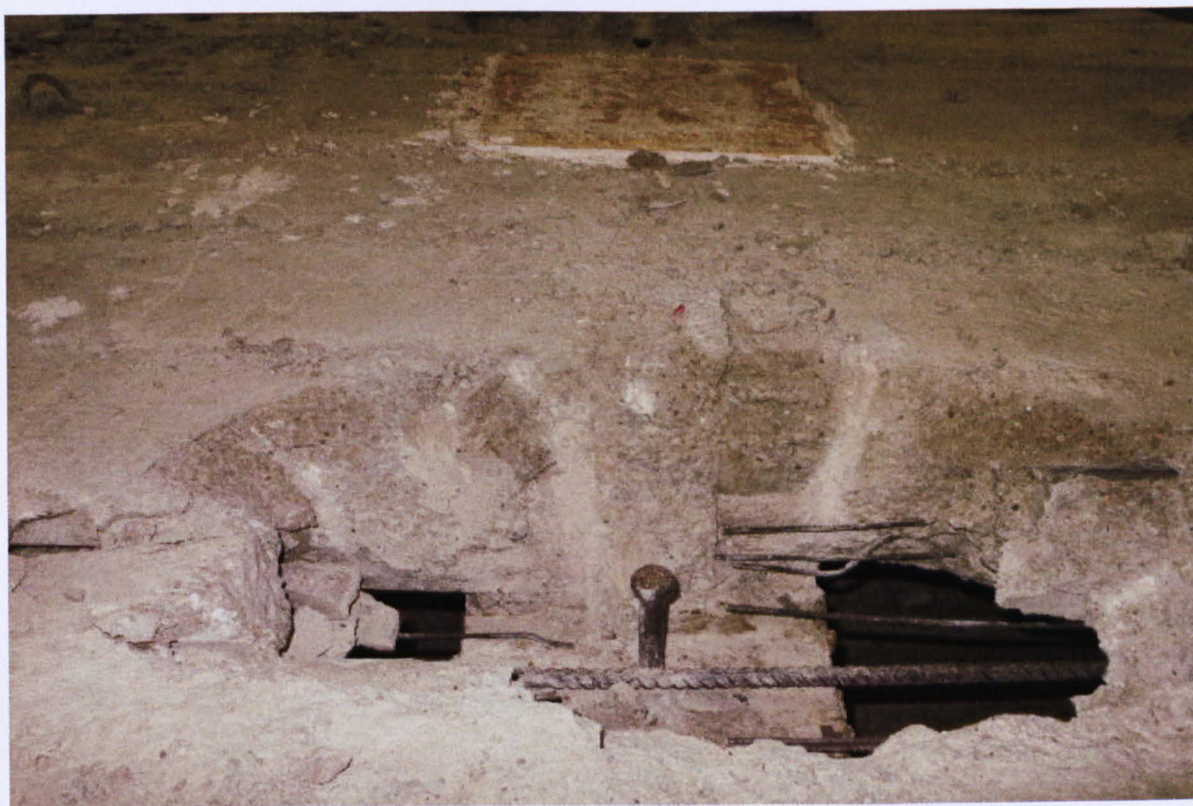
Figure 4.15: Exposed studs on South side of CB-2
