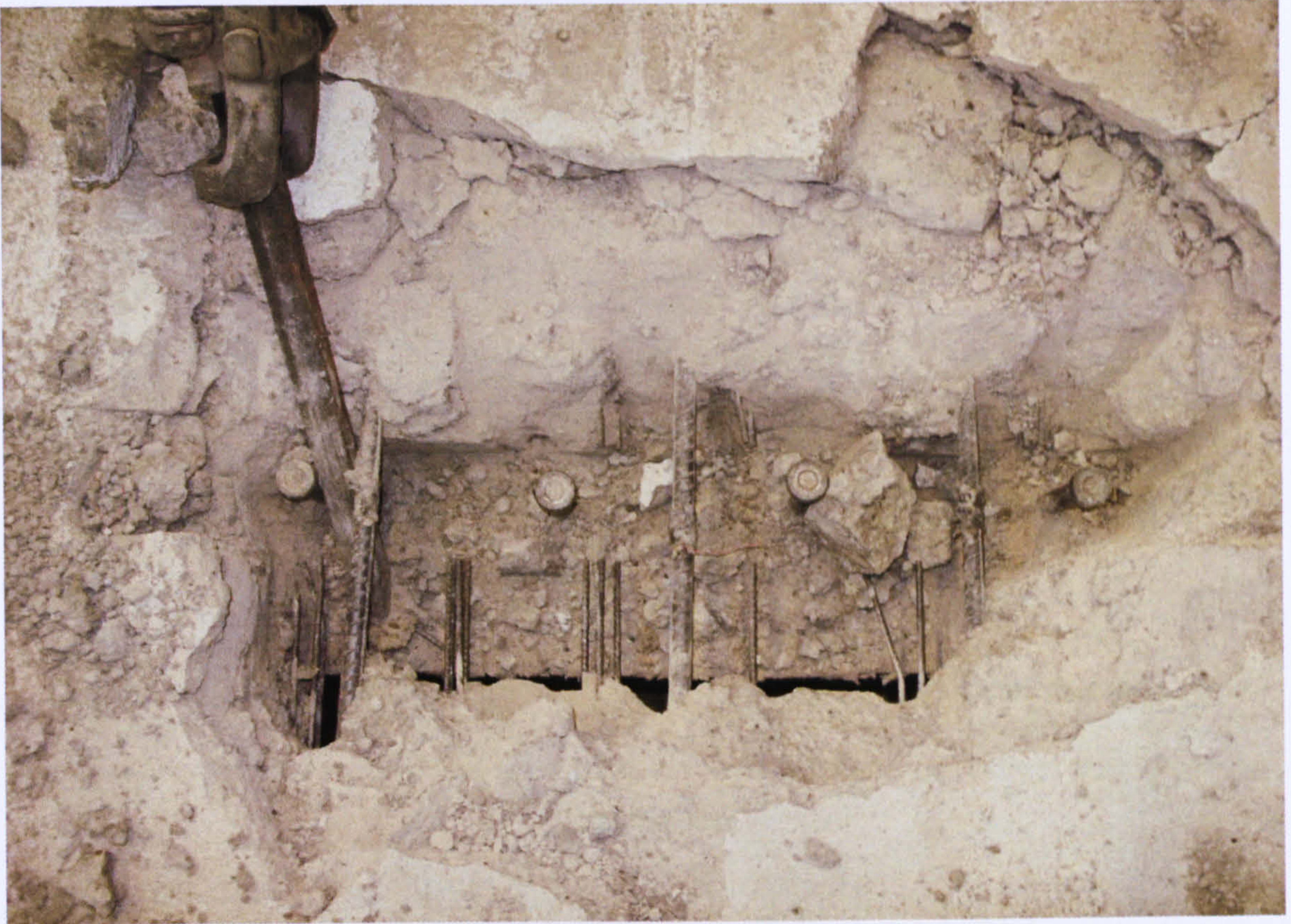
Figure 4.6: Exposed studs on North side of CB-1
