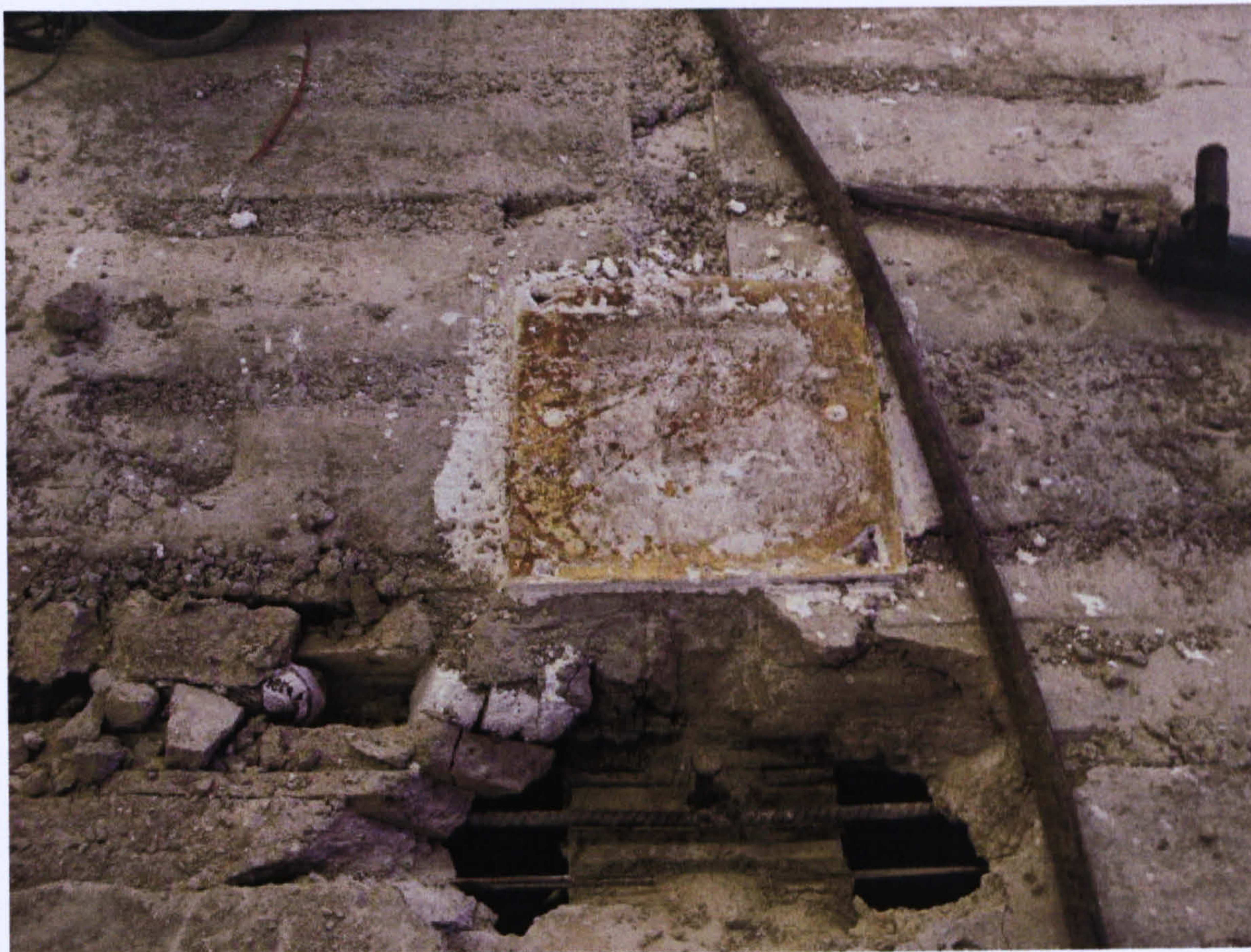
Figure 4.14: Exposed stud on North side of CB-2
