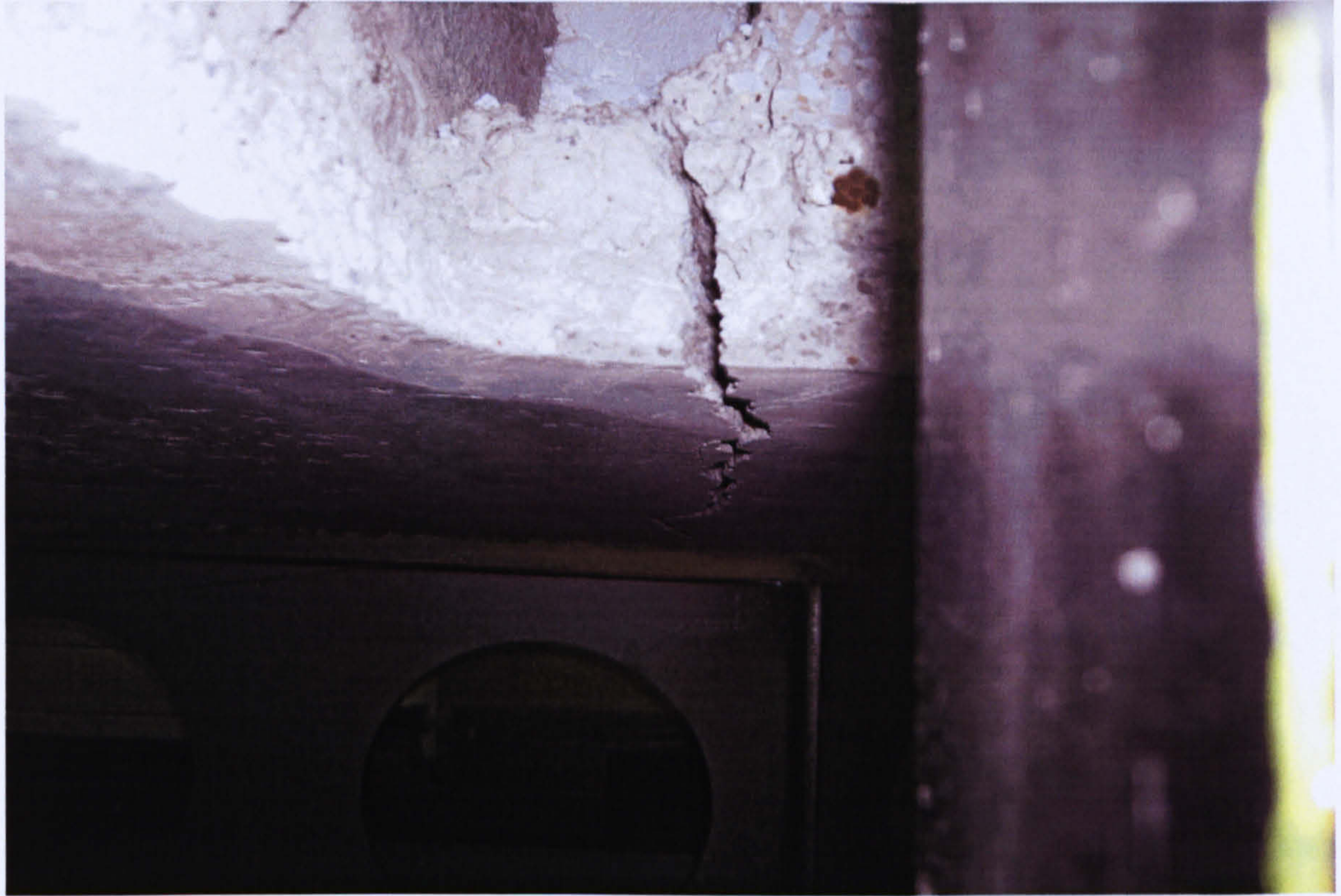
Figure 4.41: Excessive cracking on underside slab of CB-5 (West)
