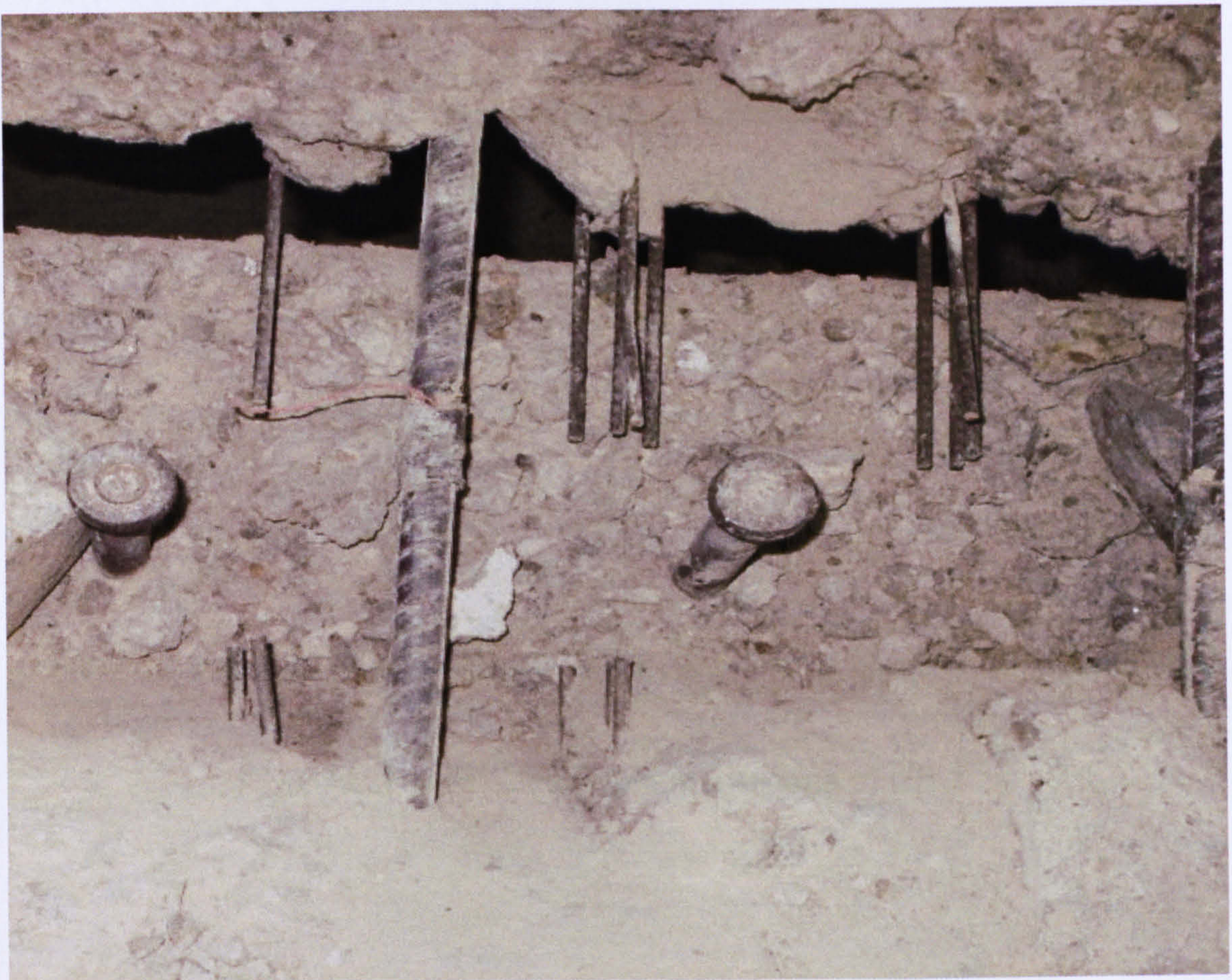
Figure 4.7: Exposed studs on South side of CB-1
