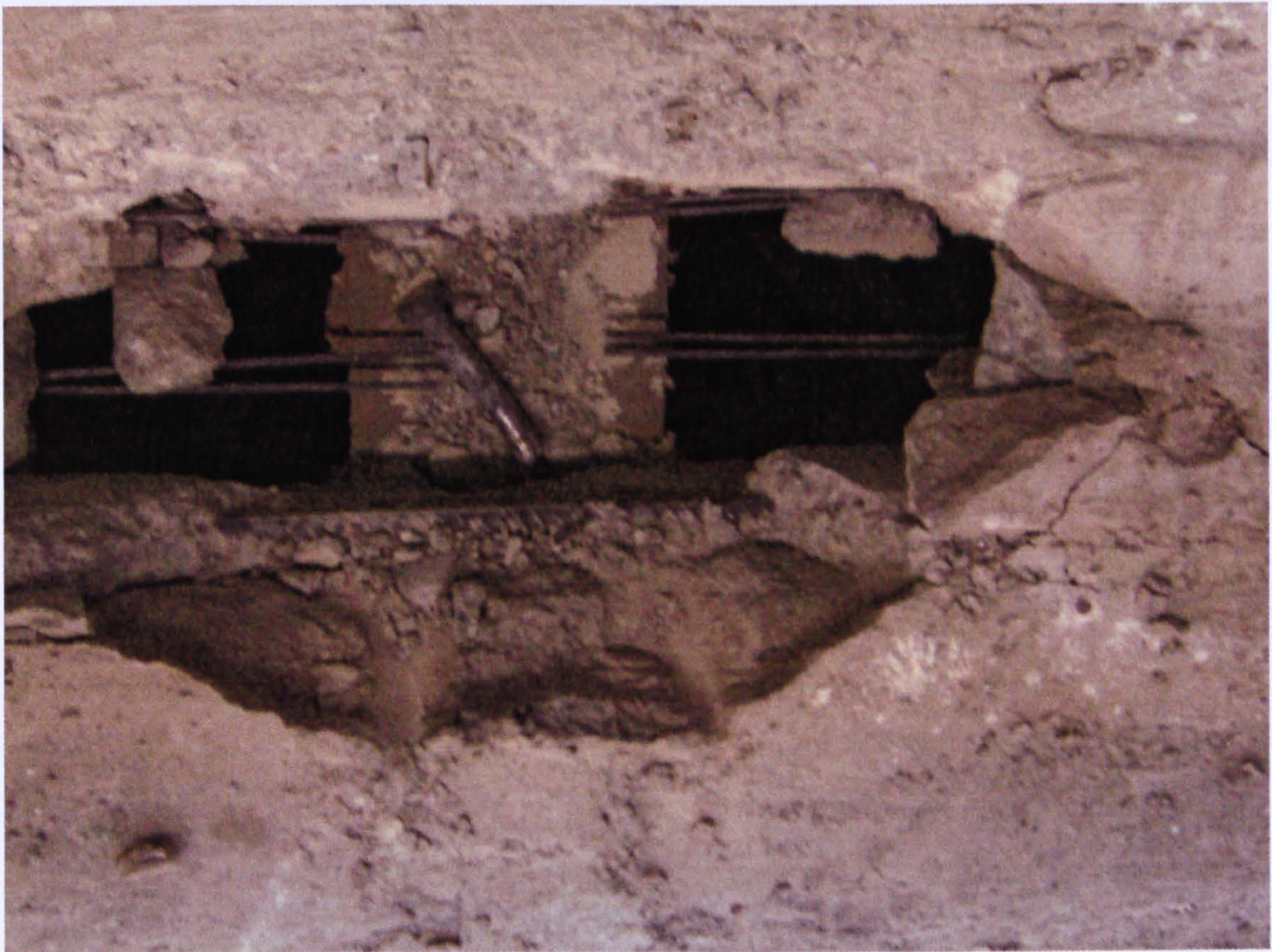
Figure 4.23: Exposed stud at mid-span region in slab of CB-3
