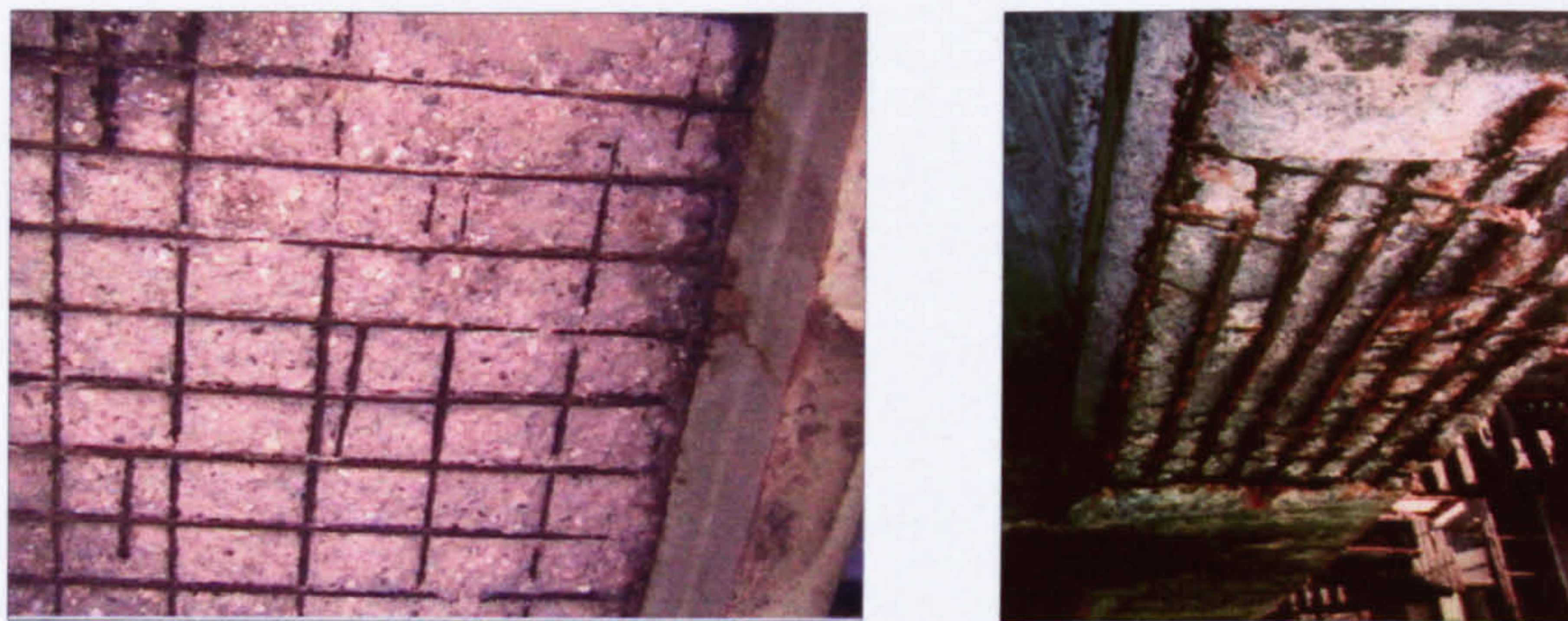
Fig. 1-1 Example of reinforcement corrosion under aggressive environments (Federal Highway Administrator 1997)
