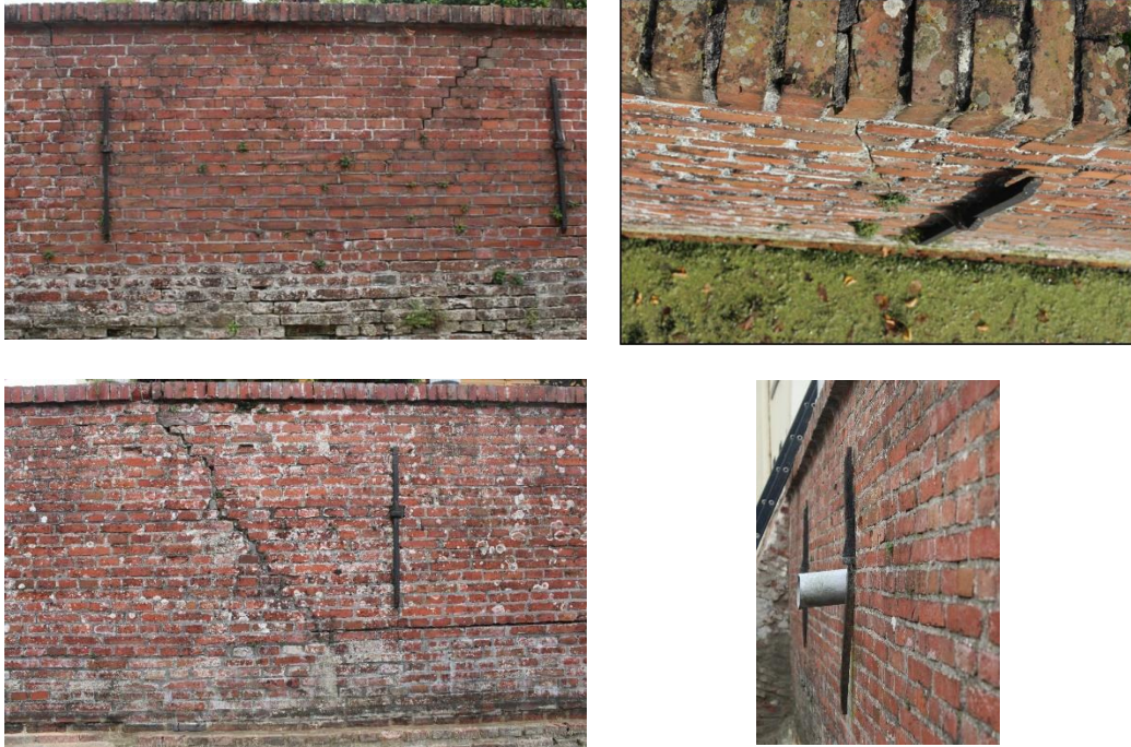
Figure 3-6: Cracks along the front retaining wall (left) and detachment of the steel anchors (right).
