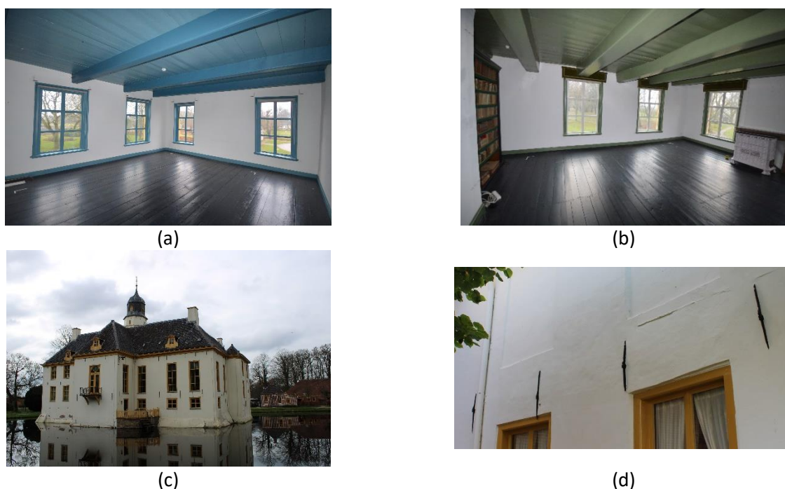
Figure 3-3: Details from the timber floors (a-b) and steel anchors (c-d) around the monument.
