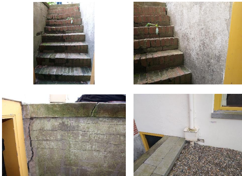
Figure 3-5: Signs of damage around the entrance of the basement located at the front NW wing.
