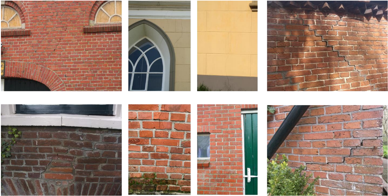
Figure 1-1: Typical examples of damage in buildings in the Groningen gas field. Photographs taken by Dimitrios Dais.
