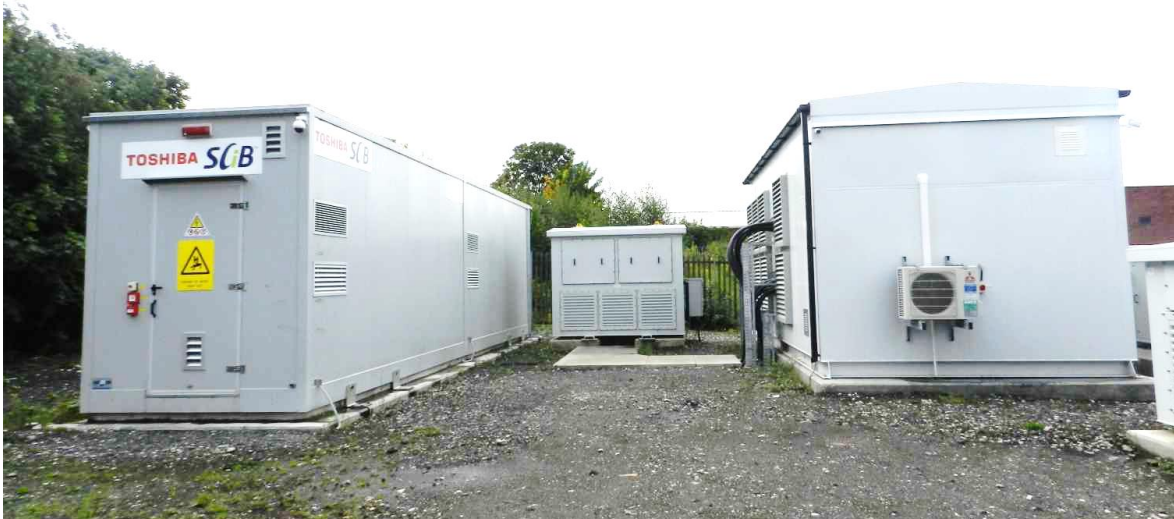
Figure 1.3 Willenhall Energy Storage System (source: [15])
