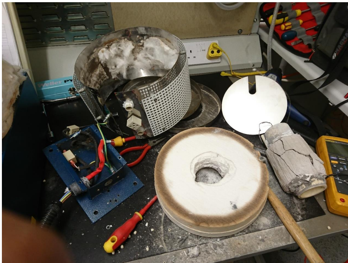
Figure 4-7: State of the furnace after a malfunction undergoing repairs.
