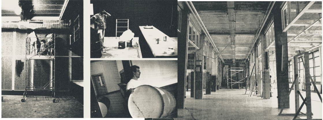
Image 6 État d'Urgence members realising renovation work inside L'Usine (Mounir et al. 2013, p.81)
