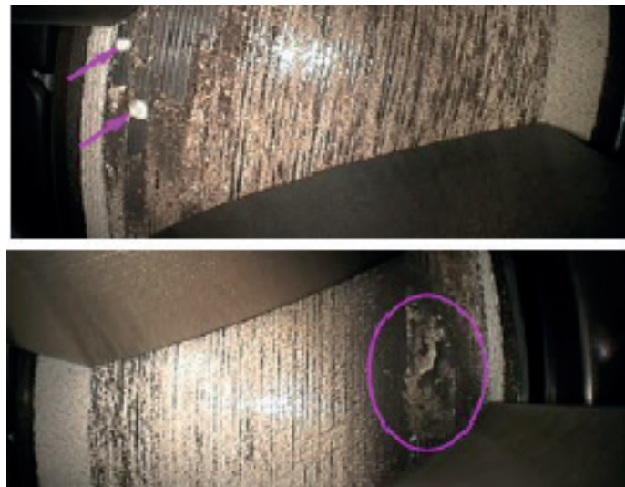
Fig. 1.13 Ceramic liner showing spallation
