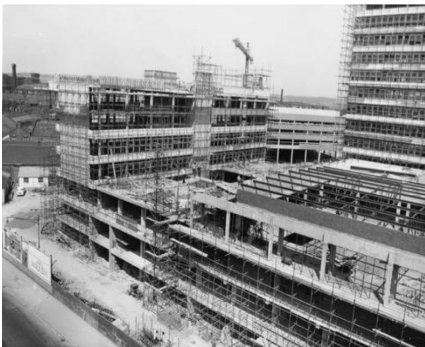
Fig 56. Town Centre Securities (TCS). c1963. Photograph of construction work at the Merrion Centre. [Photograph]. At TCS archive
