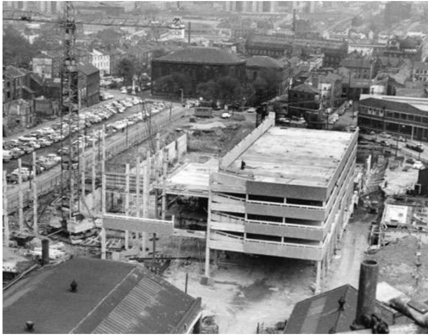
Fig 57. Town Centre Securities (TCS). c1963. Photograph of construction work at the Merrion Centre. [Photograph]. At TCS archive
