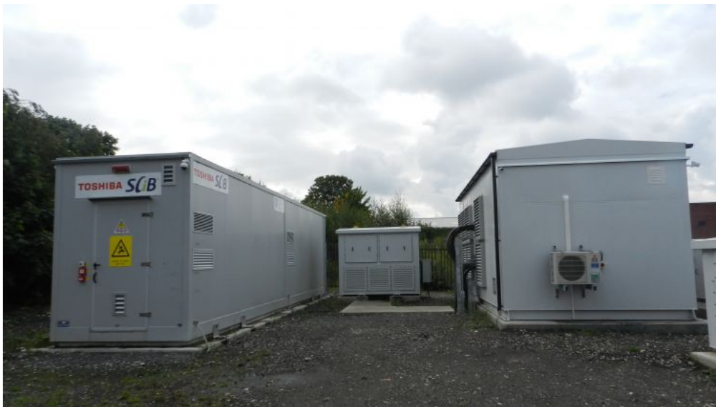
Figure 3.10: Image of the battery container (left) and inverter cabin (right) at WESS.
