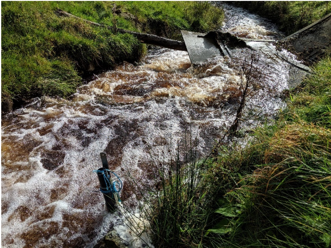
Figure B.4: Collapsed footbridge causing a backwater effect at the downstream gauge on Downs Gill
