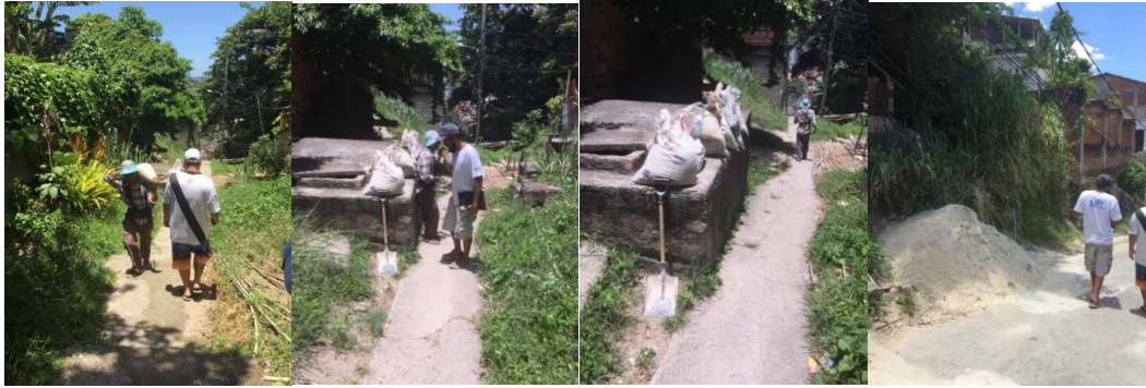
Figures 21a; b; c; d – Local residents often transport the materials on their backs, to the construction/expansion of their own dwellings. The presence of many steps throughout the pathways limits the possible help of pushcarts to specific areas.
