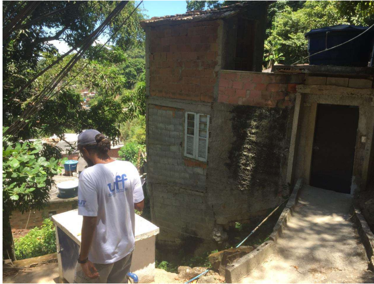
Figure 29 – Fairly uneven construction observed to the right. Only a specialist to understand the risks it poses.
