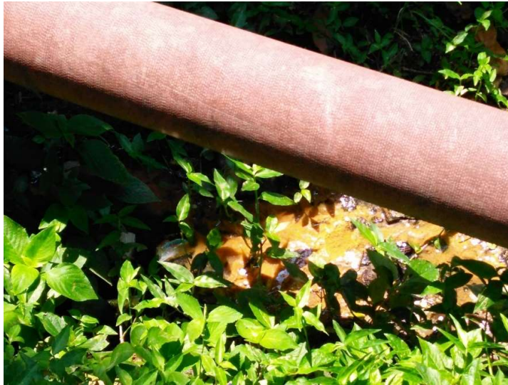
Figure 39 - On the days of the visit, it has been a while since last time rained. Some liquids that could be sewage or grey wastewater could be noticed in a few places of the community. In the cases shown in the pictures, they were adjacent to the sewage network, what could be leaks or not.
