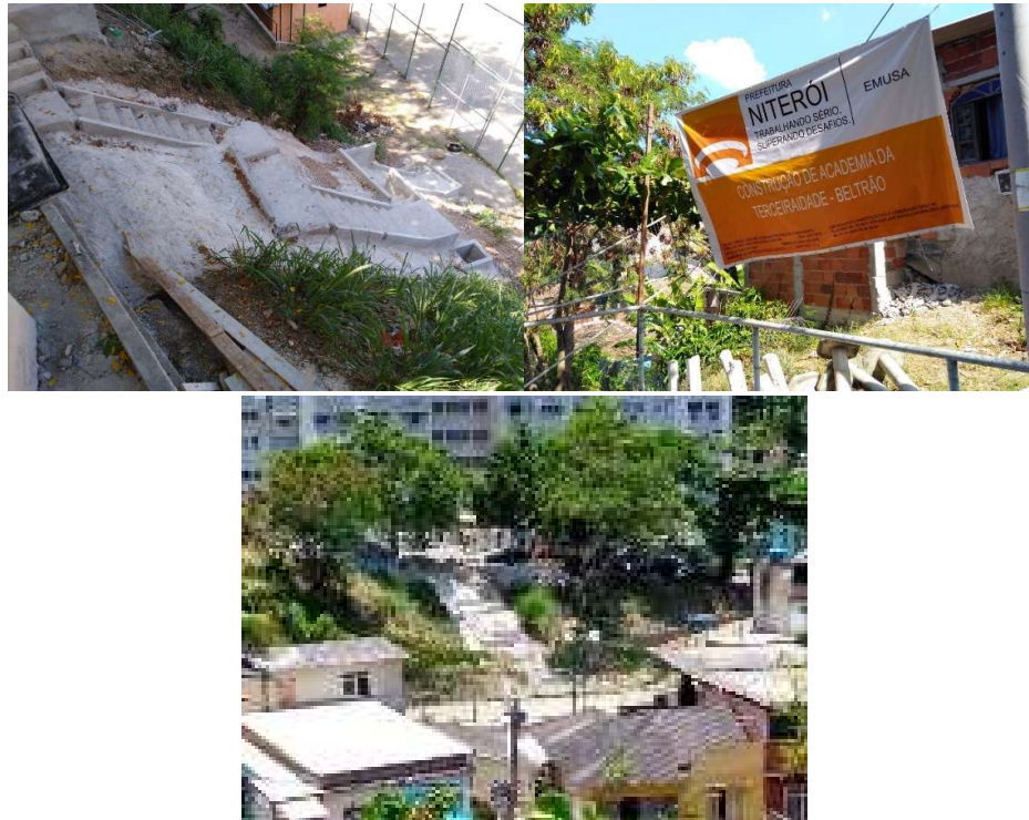
Figure 50 – City council works and the sign publicizing the construction, at the cost of 90.000 Reais, of a small space of an elderly open air gym (a few metal structures that serve as the equipment’s composes it, and its accompanied by 3 concrete tables with 4 benches). Despite being an intervention made for the public common use, Local residents commented it was never a demand from the community, but the local resident association played its part on “accepting” the investment. It could be tried to reach the stakeholders, in this case the city council to know if there is any sort of technical material that could serve for a quantification of the materials used in this public intervention also.
