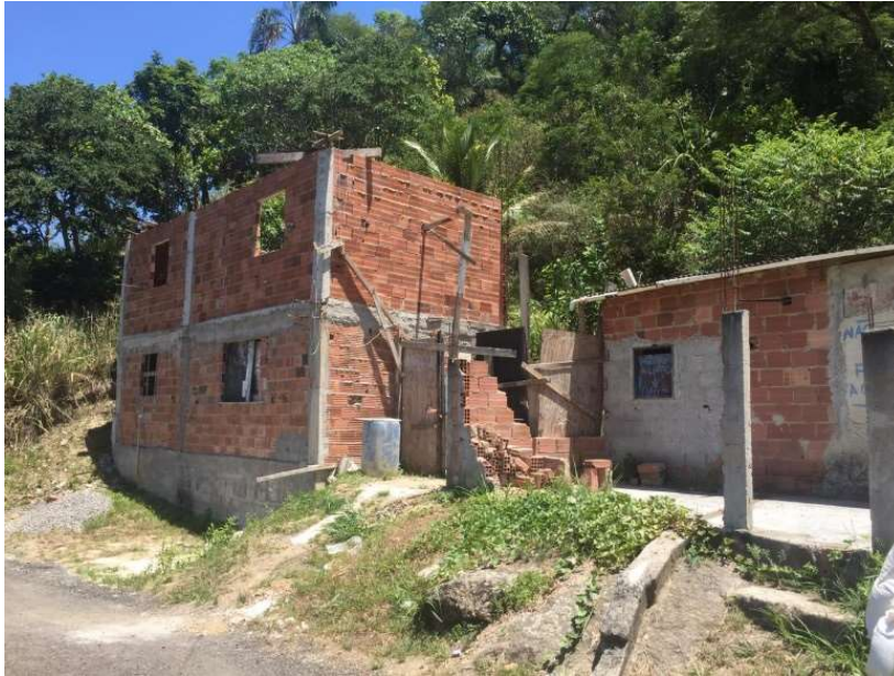
Figure 37 – Next to the local resident that have a house under construction (a). He was the one that informed that the houses of this upper location do not have water reaching through the network. On the back, the 8000 litres water-tank that he was fixing the leaks and connections to receive the water-tank truck. This is a fair example of the sort of information that is impossible to be obtained without reaching the local residents.
