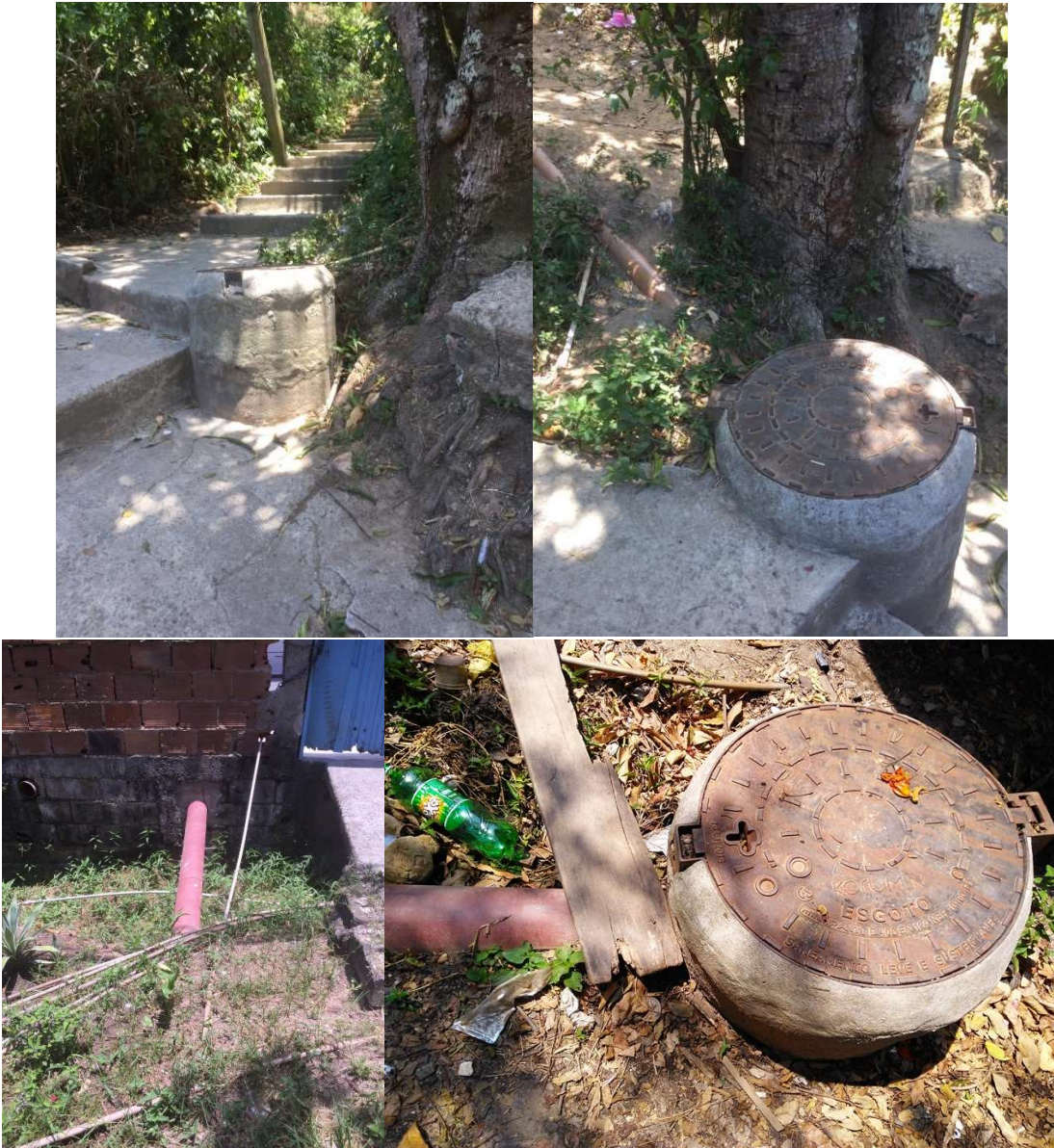
Figure 38 - Recently installed network, the works were done only in 2017. New residents than have to connect their houses to the network themselves. It could be explored what are the obligations of the stakeholders in this case, and what are the limitations for the expansion and inspections of the sewage disposal in these places. The problems of being formally recognized or having or not land tenure rights, should not be an excuse for not dealing with the environmental problems that are happening independent of social or political disputes.
