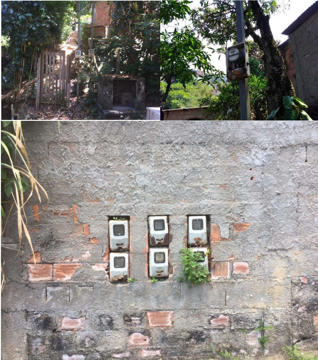
Figure 42 - Old rusty energy meters. They are all over the place, besides the comments that no one paying energy. This element and its physical and temporal connections can be further explored in the research.
