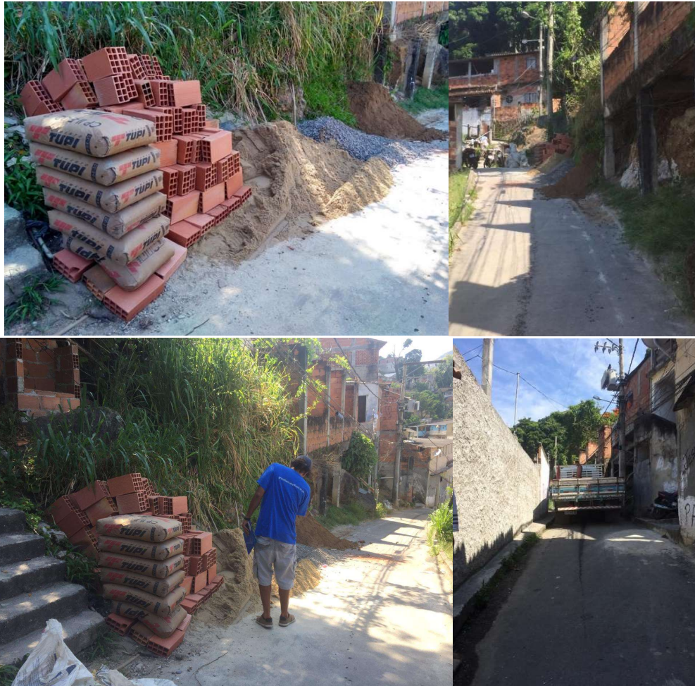
Figures 20a; 1b - Construction materials stored at the furthest point that a truck can reach in the informal settlement. From this point, materials are transported by hands to the locality of the construction.
