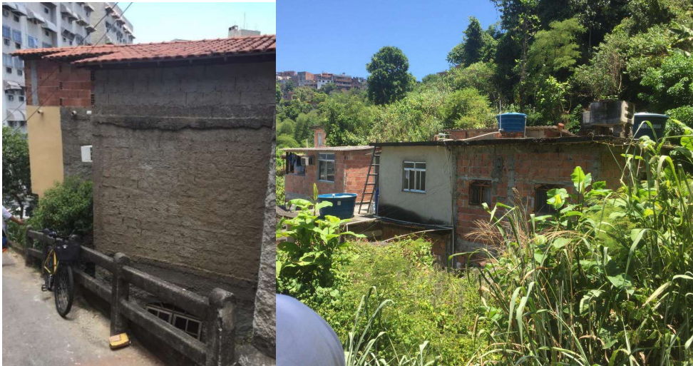
Figure 24 – Different courses of outside walls finishing side-by-side on the same geminated constructions. Even including exposed bricks, there seems to be no defined rule when it comes to considering a house as finished or not.
