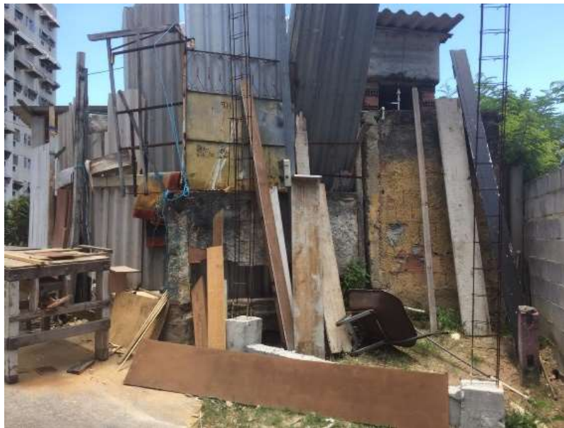
Figure 25 - An extension of the house under construction. According to the resident, it had to be given up, due to losing his job and getting into financial hardship. The construction materials have been stock in an improved way, creating risks for the surroundings and his own safety.
