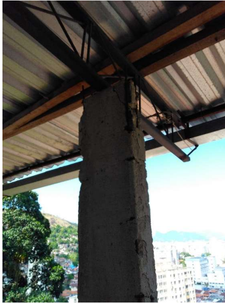
Figure 31 – Some building pathologies are noticed as the construction processes, frequently lack quality control and can be even done in an auto-constructed auto-didactic way.
