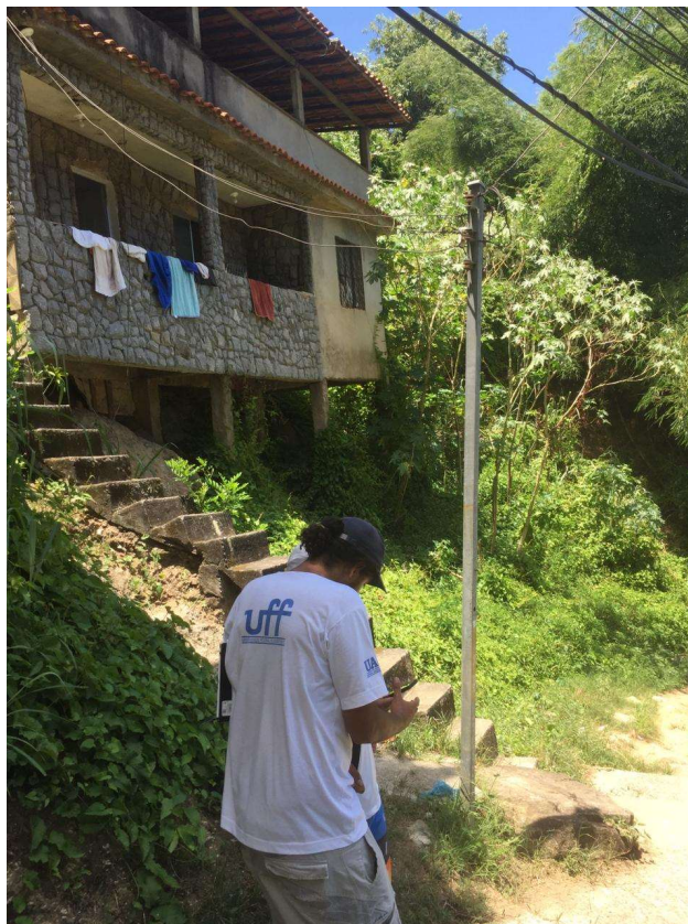
Figure 27 - On the back, a house that has been condemned by the state civil defence specialists. Residents still live in as evidenced by the clothes drying in daylight. Columns on the bottom that sustains it looks worryingly bent, and as it can be seen, the house is made of stones certainly adding too much weight to it. At this point Rafael, we were facing, and he was explaining where and how the house he lived went down on the landslide 10 years ago.
