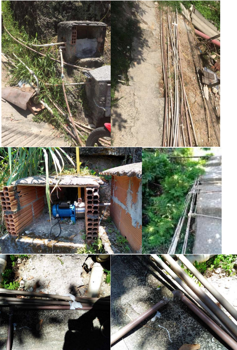
Figure 34a; b; c; d; e; f - Water infrastructure elements installed to the formal network of the water services providers (Águas de Niterói). The hydro-pumps (a; c) belong to the residents. The fragility of the superficially exposed system that connects the pumps to the dwellings is evident in the other pictures and it's possible to observe numerous repairs.
