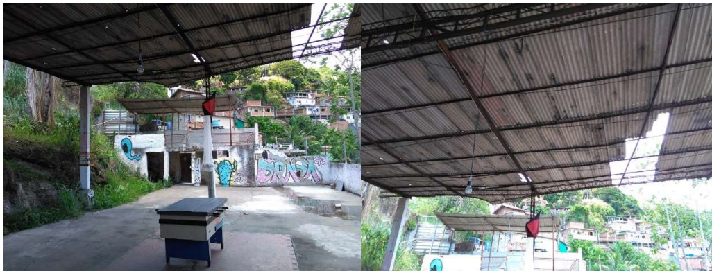
Figure 49 – The local “quadra” (court), a public space where a bar is located and historically, gatherings used to happen for leisure in the nights and weekends. Due to the risks posed by bad state of conservation of the roof the frequency of costumers is not the same, rendering less useful this common space of interactions between the residents.
