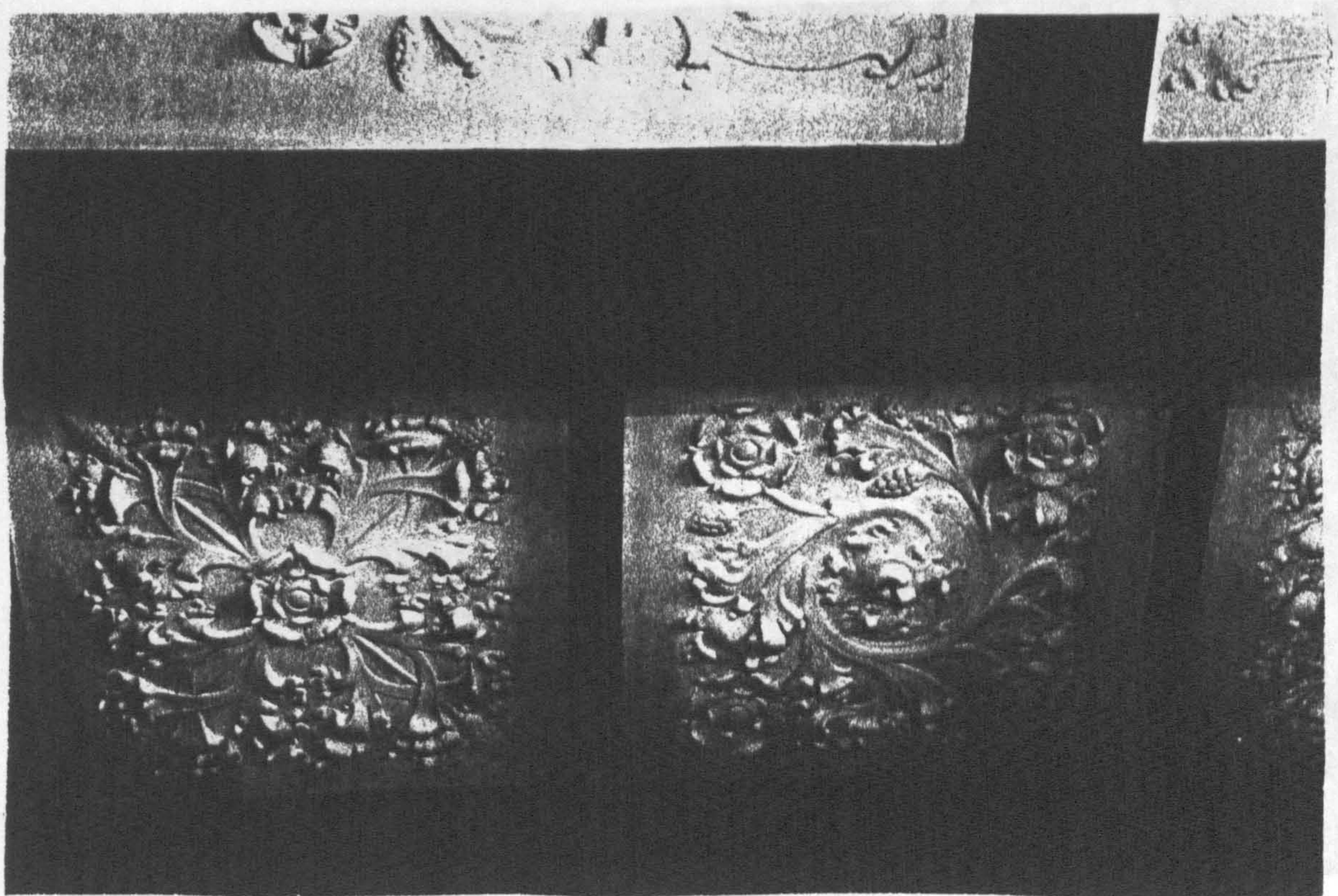
3/31: Plaster ceiling decoration, John Rylands Library, Deansgate, Manchester. (Architect, Basil Champneys) 1899. (Auth) [cat 117]
