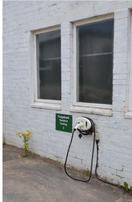
Figure 4-64. Electric vehicle charging point
