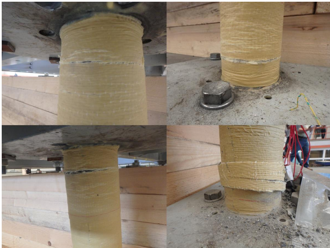
Figure 5.14: Rupture of the AFRP jacket of the base-isolators after the 2.0g PGA test
