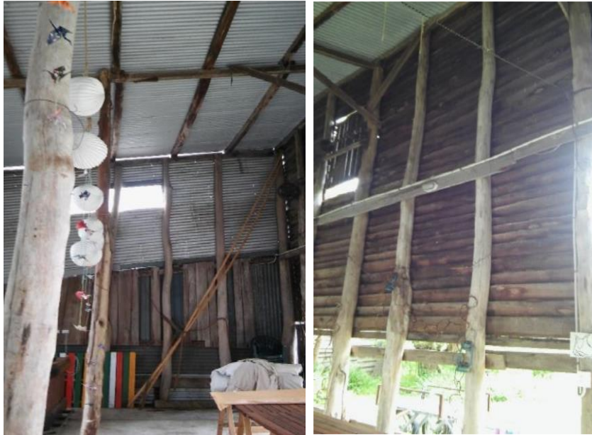
Figure 22: Old shearing sheds. Vernacular architecture invoking colonial nostalgia, Fairharvest farm. Photograph by author Oct 2017
