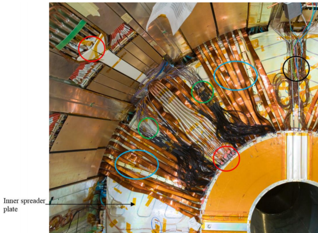
Figure 28: Photo of the ID barrel services with the cover removed, taken from [88]
