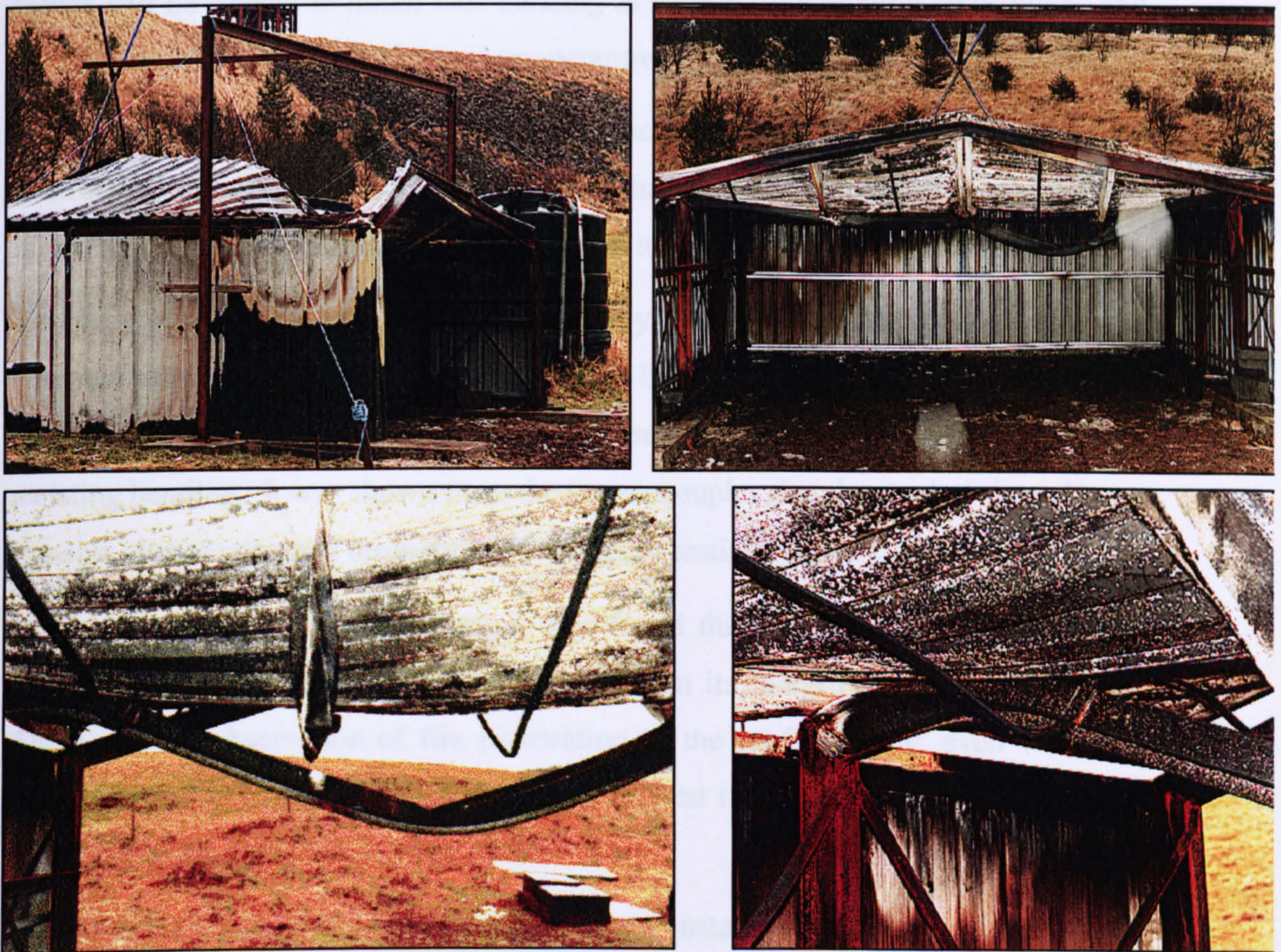
Figure 4.27 Collapse of the portal frame (top) and fire hinges formed during the test (bottom)
