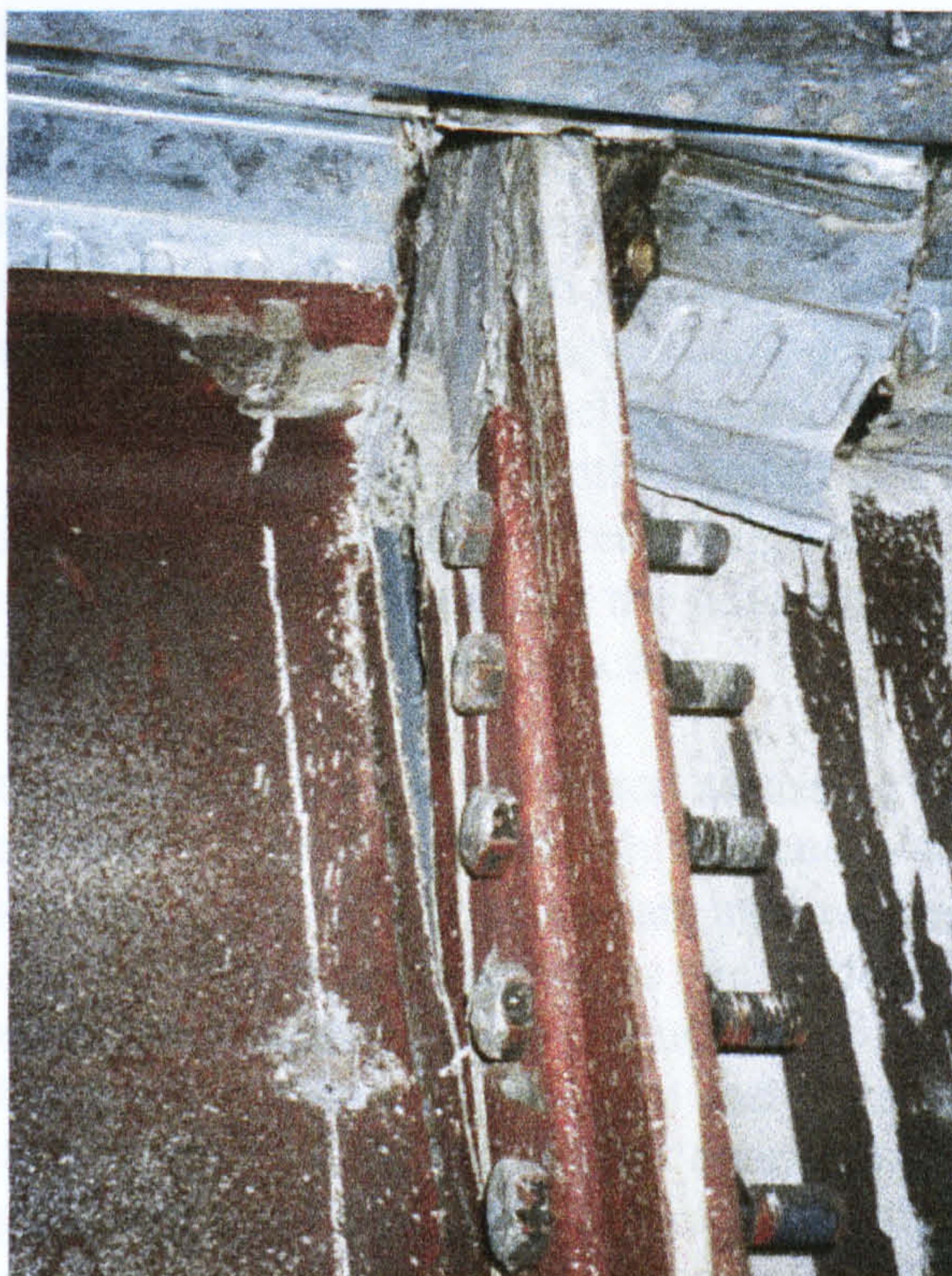
Figure 4.17: Elevated Temperature End-Plate Failure Mode for Group 5
