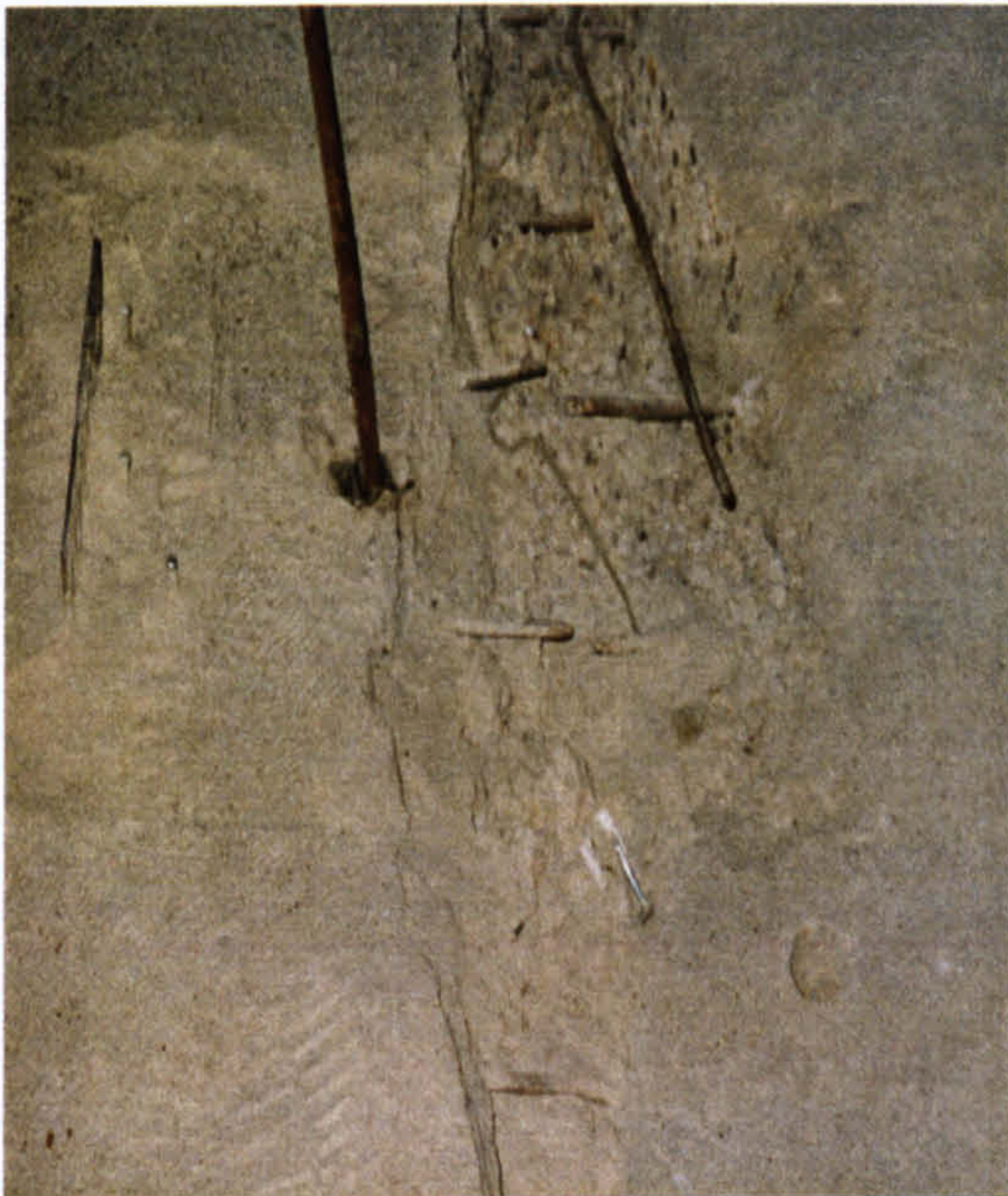
(a) Slab Cracking and Fracture of Bars
