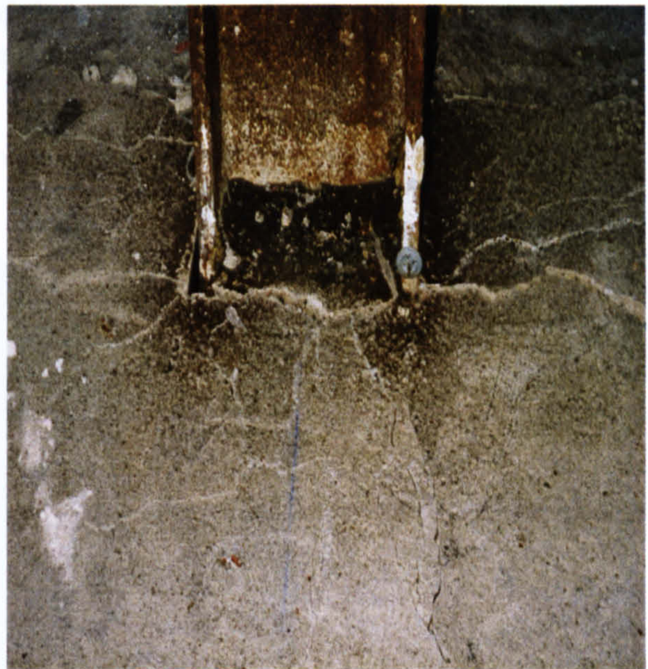
(b) Cracking Patterns around Column
