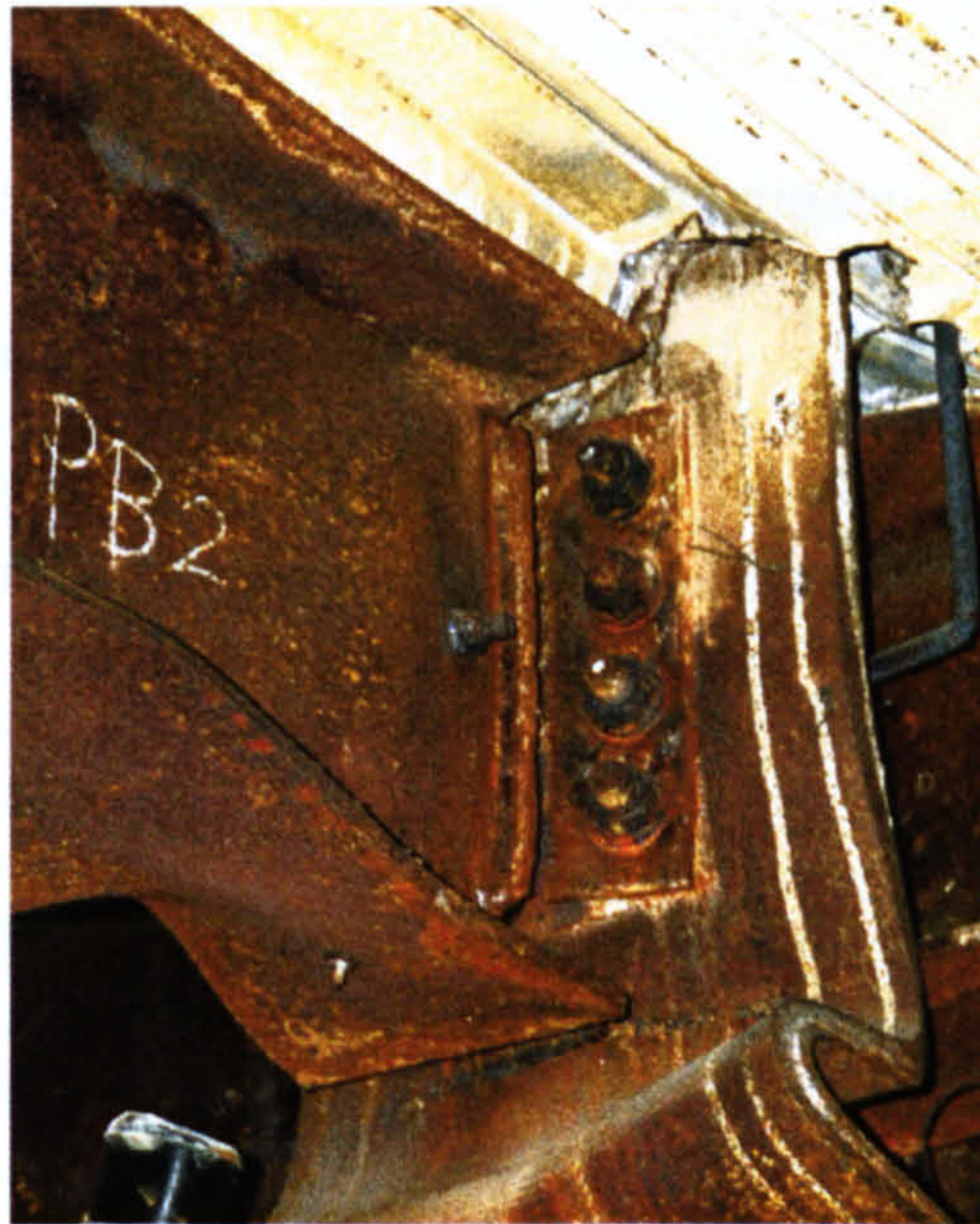
Figure 6.23: Local Buckling of Beam Flange and Exposed Column Zone in Cardington Tests
