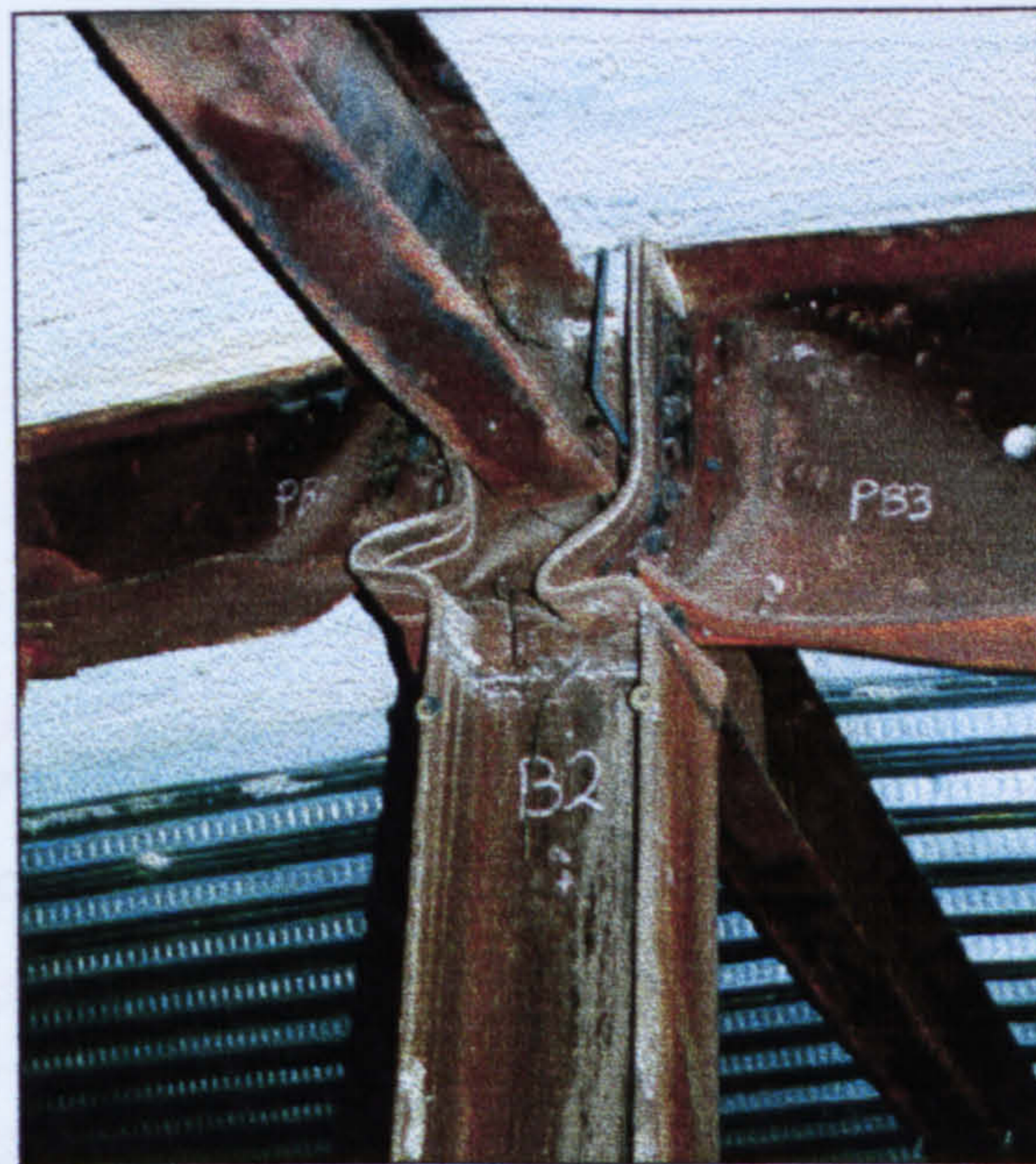
Figure 2-12. Photograph of the head of buckled column on gridline E2
