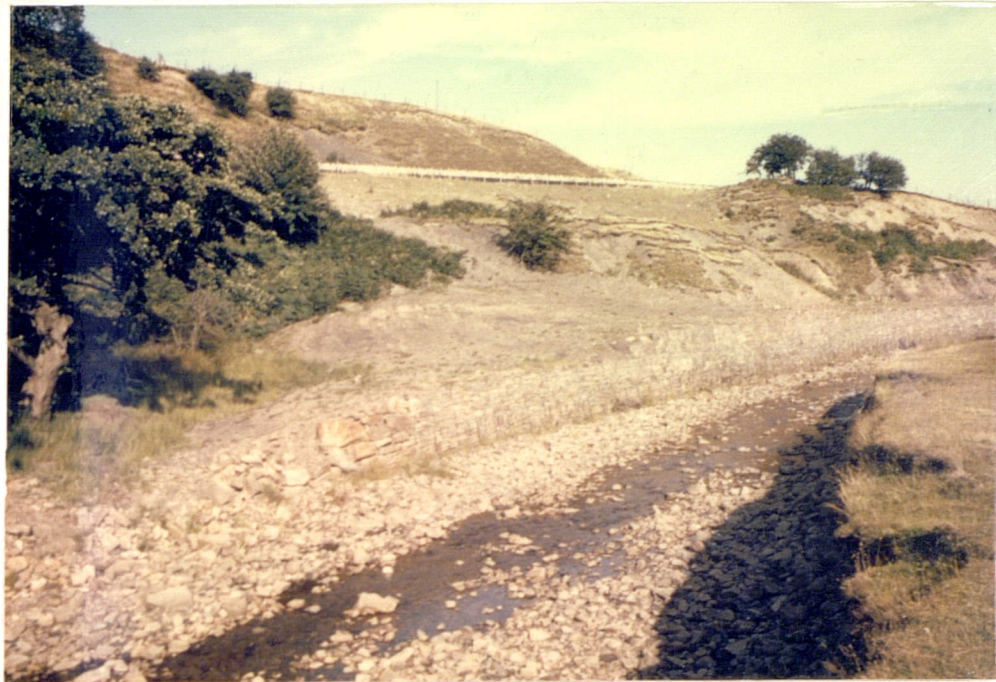
Plate No. 7.48 Gabbion wall to protect the toe of the landslip at Rowlee Pasture.
