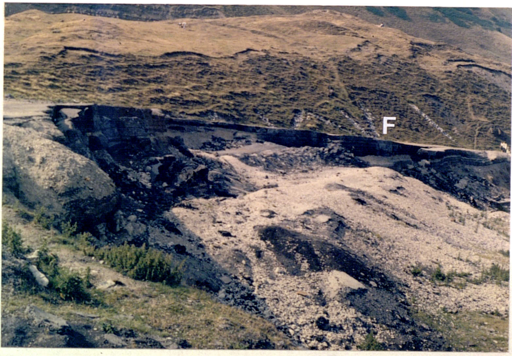
Plate No. 7.5 Damage at the upper road at Mam Tor. Note that successive layers of road surfacing material have been applied in an attempt to maintain the road. French drains on main unit of Mam Tor landslide 'F'.
