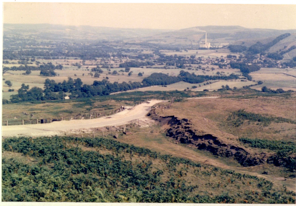
Plate No. 7.9 Heave movement at northern part, Lower road.
