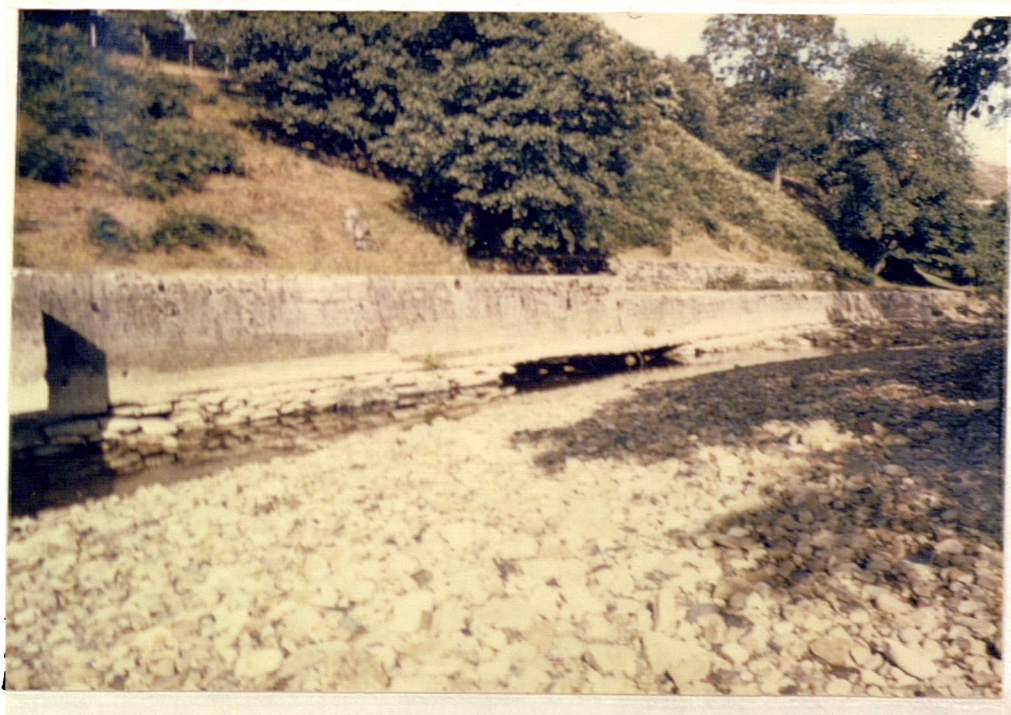
Plate No. 7.49 Concrete wall to protect the toe of the landslip at Rowlee Pasture.
