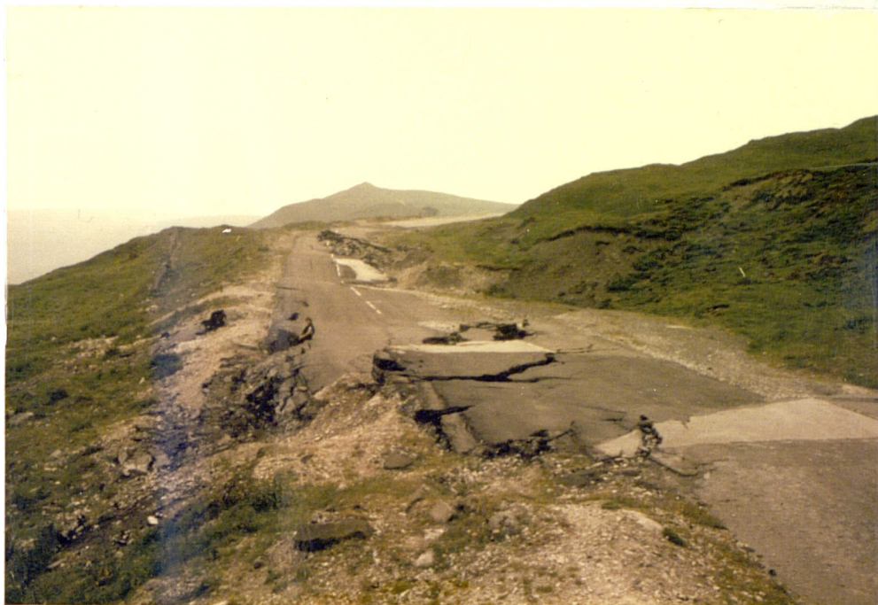
Plate No. 7.6 Damage of the upper road at Mam Tor. Note that the recent instability has caused a downward movement with lateral displacement.
