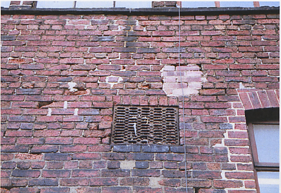
Fig. 2.92 Detail of the side elevation, above, with an original ventilation grille from the back wall of the grinding hulls. Note the later window to the right (author).
