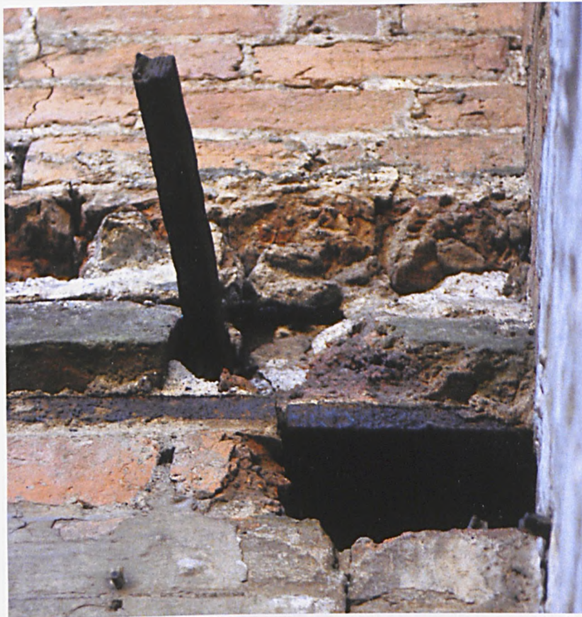
Fig. 4.96 Projecting tie rod that connected lateral iron beams and counteracted the outward thrust of the vaults, with the flange of an embedded 'T' beam visible beneath (author).
