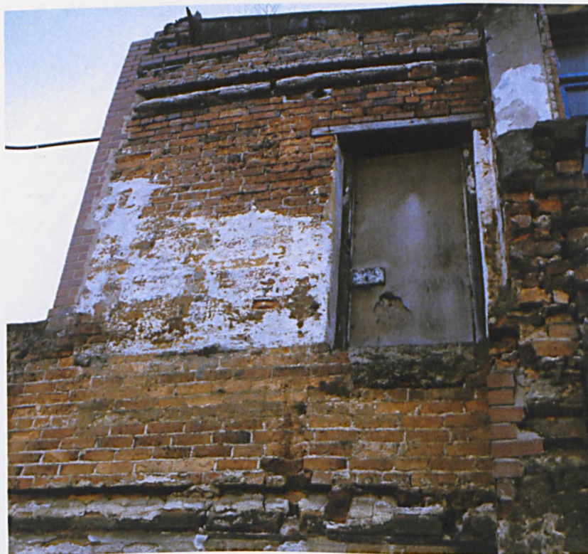
Fig. 4.97 Looking up to the first and second floor springing structures. The third floor would have been constructed of timber boarding (author).
