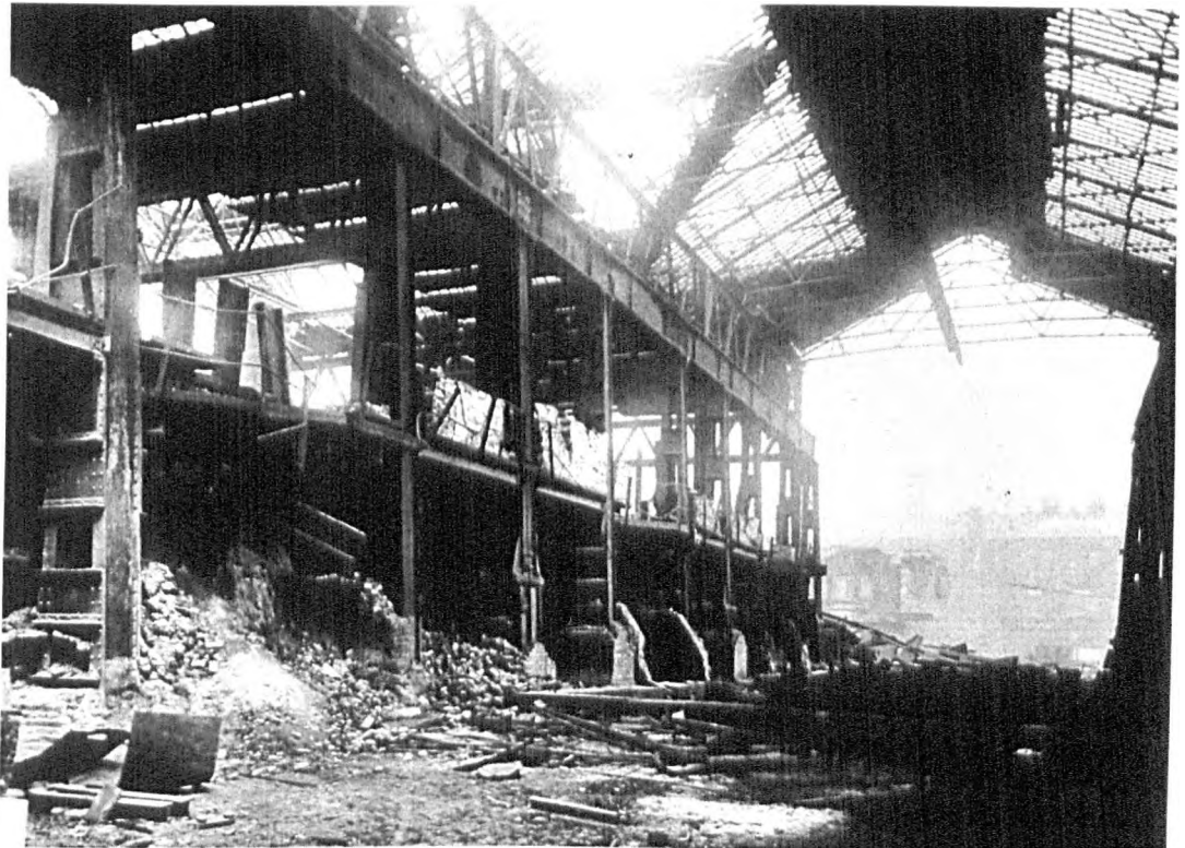
Fig. 5.70 Photograph inside the steel melting shop during alterations. The heavy masonry structures at basement level may be the remains of the original crucible furnaces (SCL).
