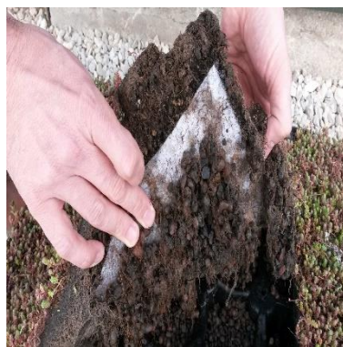
Figure 7.23. Example of a sedum vegetated green roof system that roots system reached drainage layer (Source: https://www.gtspecifier.co.uk/green-roofs-living-walls/green-roof-garden-vegetation/sedum-green-roof-trays ).
