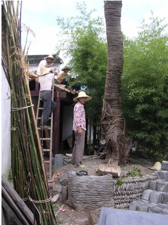
Figure 5.12 A new garden in Hongcun under construction on the location of an orchard. This was said to have previously been a garden, but few historical features had survived. The craftsmen who constructed this came from neighbouring villages and their techniques reflect vernacular construction methods. For example, the raised bed under the tree was encompassed by pebbles from the riverbank in the village, and was constructed in the same way as the traditional drainage ditches in the village. (Source: photo by author, August 2007)
