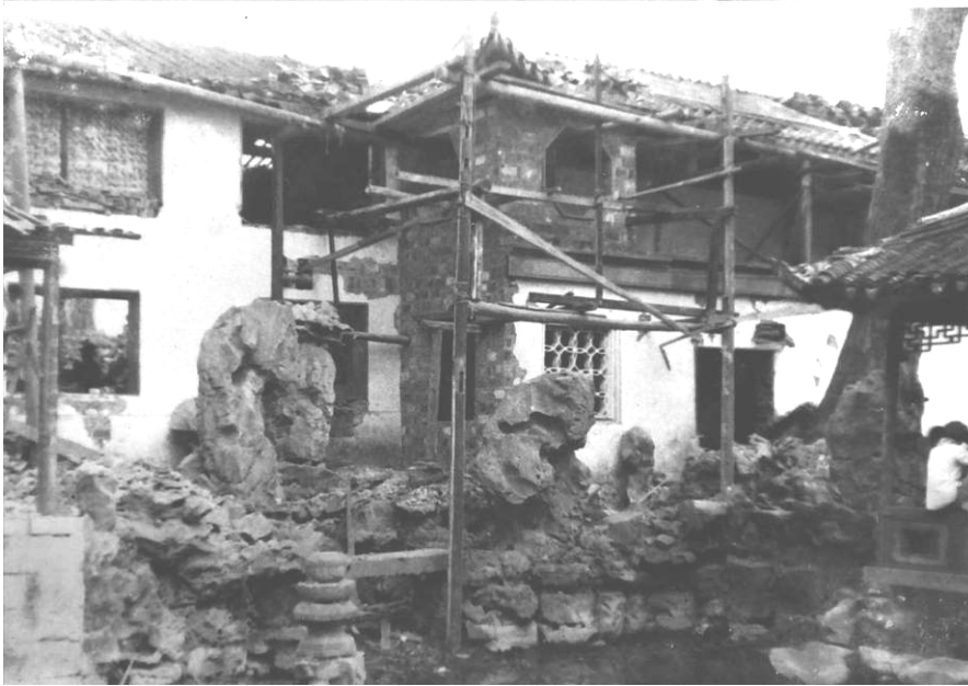
Figure 4.14 Quxi Lou (曲溪楼 Crooked Brook Tower) in restoration (1953) The building structure has been mostly well kept, but there was damage to both walls and roof, and timber window frames are missing. Other garden features such as rocks, pond, bridge and old trees are well preserved. (Source: provided by Fengquan Chen (陈凤全))
