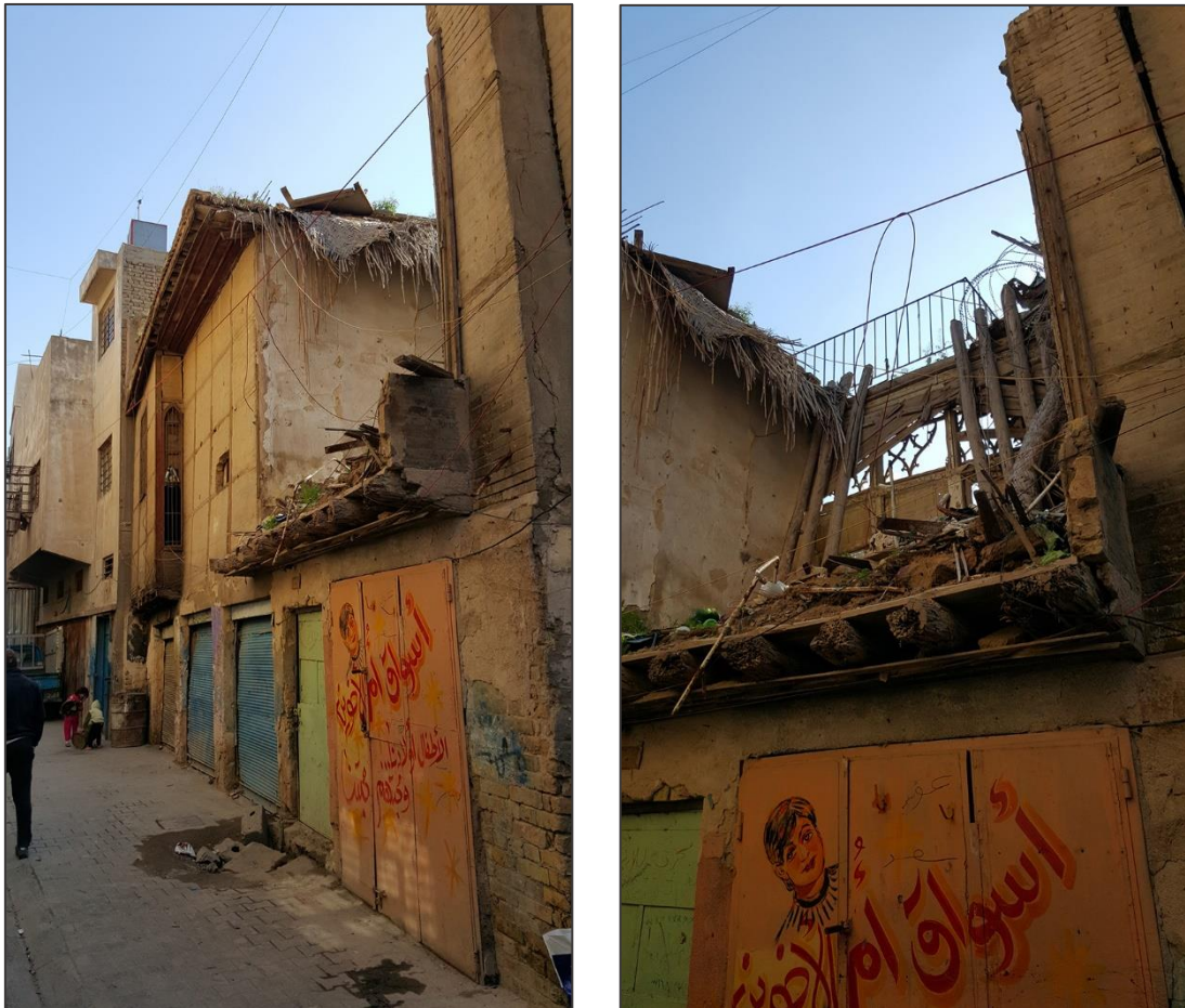
Figure 5.21-22: Baghdadi traditional house, the demolition of the roof while maintaining commercial activity in the ground floor.
