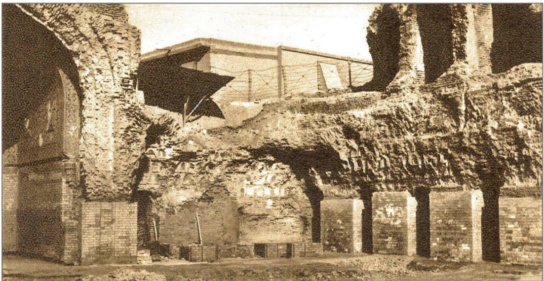
Figure 4.13: View of the intersection of the eastern and the southern wings after the first stage of intervention. 81
