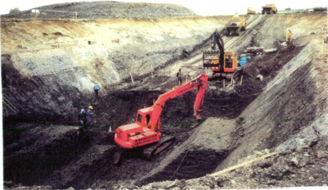
Figure 3.20 - View from south-west showing excavation from 7.5m to 10m around instrument locations (30 April 1987)
