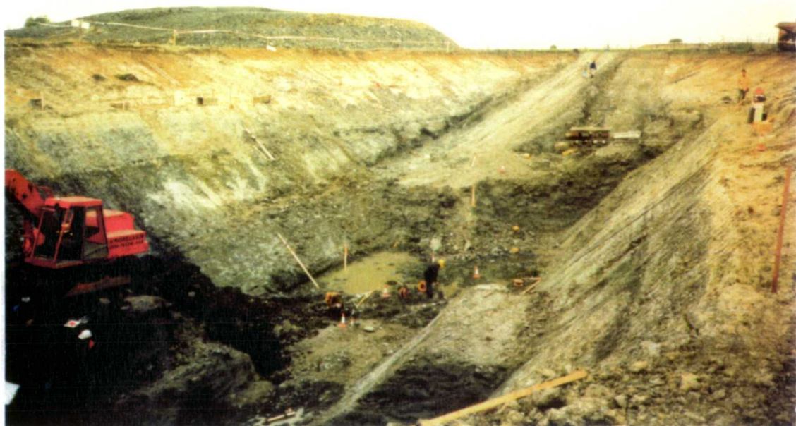
Figure 3.21 - View from south-west showing stage of excavation at suspension of works and trial embankment in background (5 May 1987)
