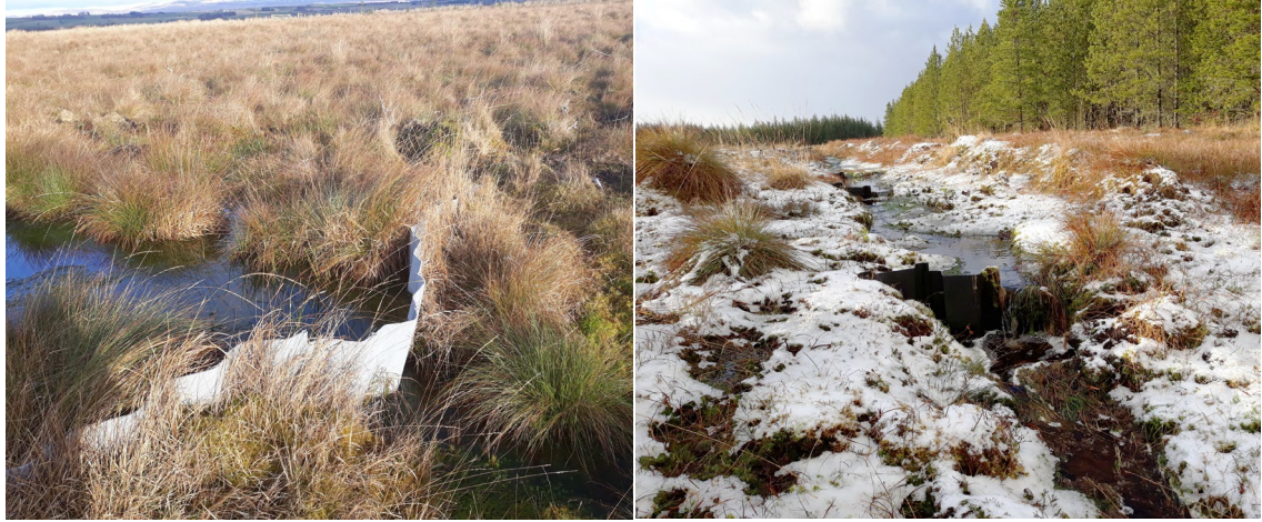
Figure 1-9 – Use of plastic piling dams to attenuate runoff and raise the water table (Flanders Moss NNR, left; Forsinain (BBR2), right).
