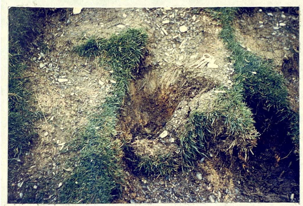
PLATE 6 Collapse of a turf step on the new path at Hawse End
