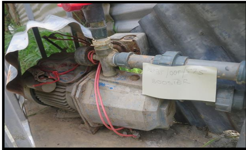
Figure 4.7: An example of electric booster pump used by some households
