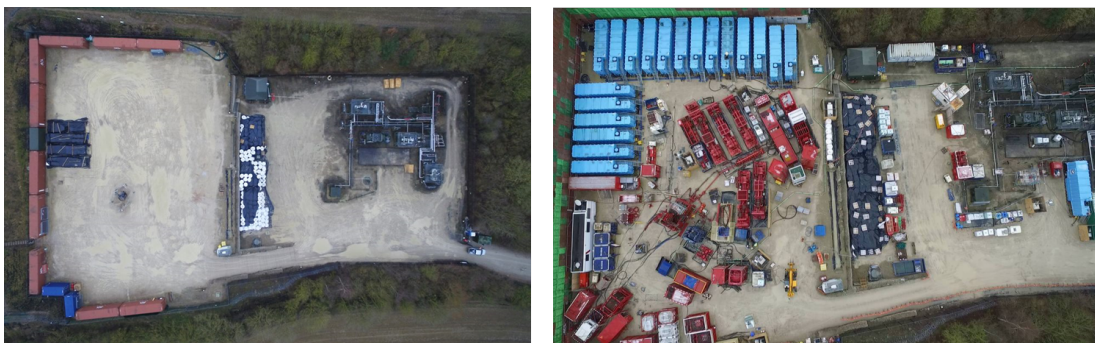
Figure 5.2: Aerial images of the Third Energy well site in April 2018 once fracking activities were halted (left) and December 2017, showing the extra equipment brought onto the site during the pre-operational period (right).
