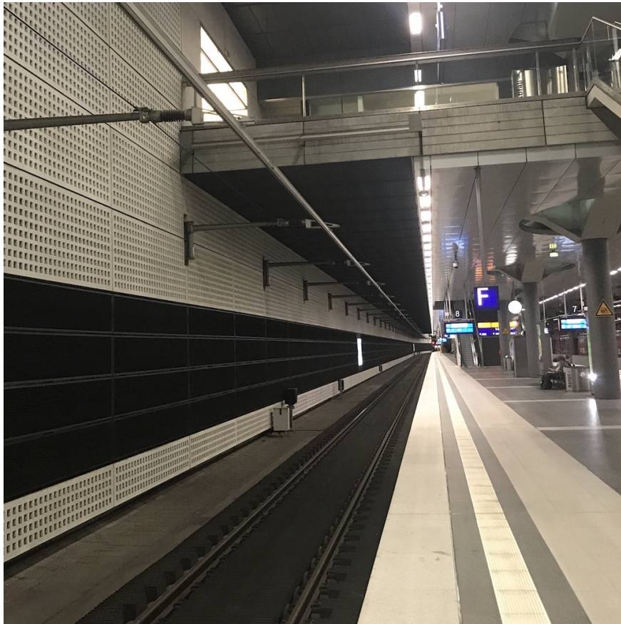
Fig. 2.11 Overhead conductor rail installed in Berlin Hauptbahnhof, Germany.
