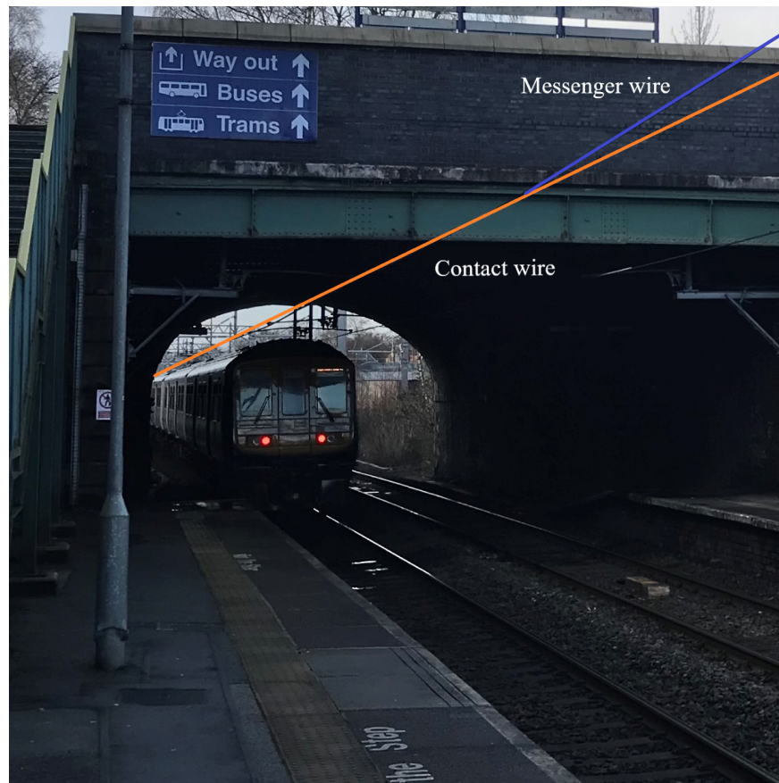
Fig. 2.9 Overhead line equipment passing under a bridge in Eccles, UK. The messenger wire height is highlighted indicating the reduction in system height to satisfy clearances.
