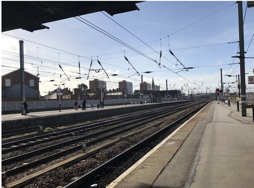
Fig. 2.7 Simply sagged overhead line equipment supported by headspans, Doncaster, UK.
