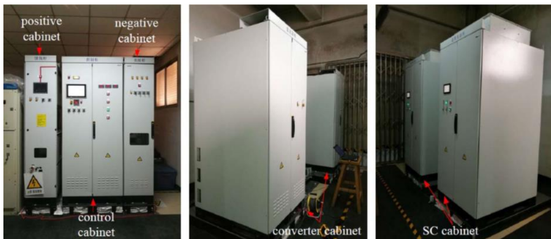
Figure 2.10: 1 MW supercapacitor system at Liyuan substation of Batong Line of the Beijing Metro, China [92]
