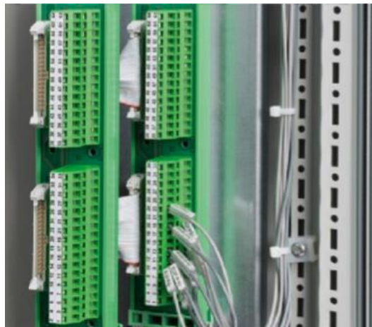
Figure 6.17: The terminal module cabinet [149]
