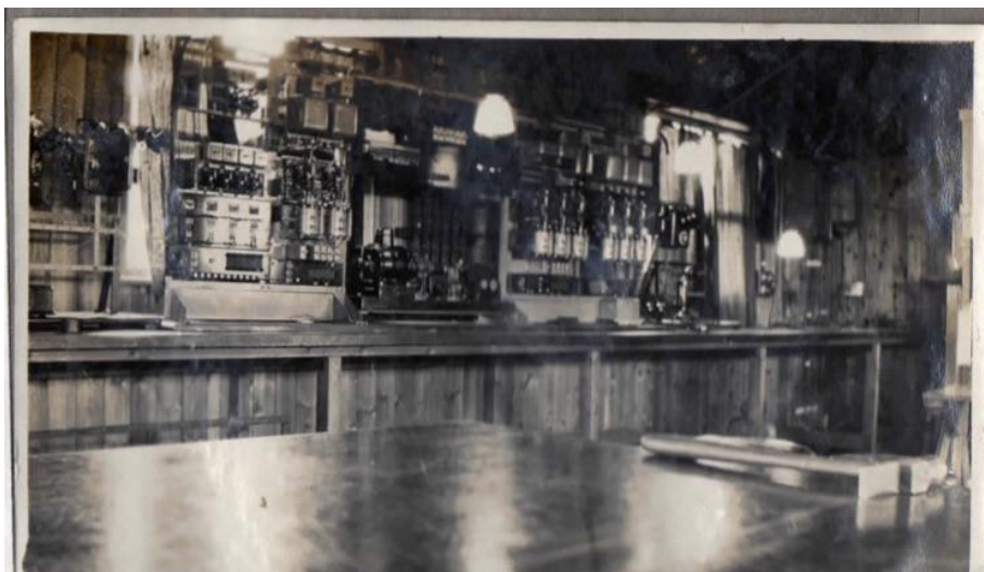
5.4—Photograph of the interior of one of the huts showing a rack of uniselectors and relays (image courtesy of Peter Belcher). 64
