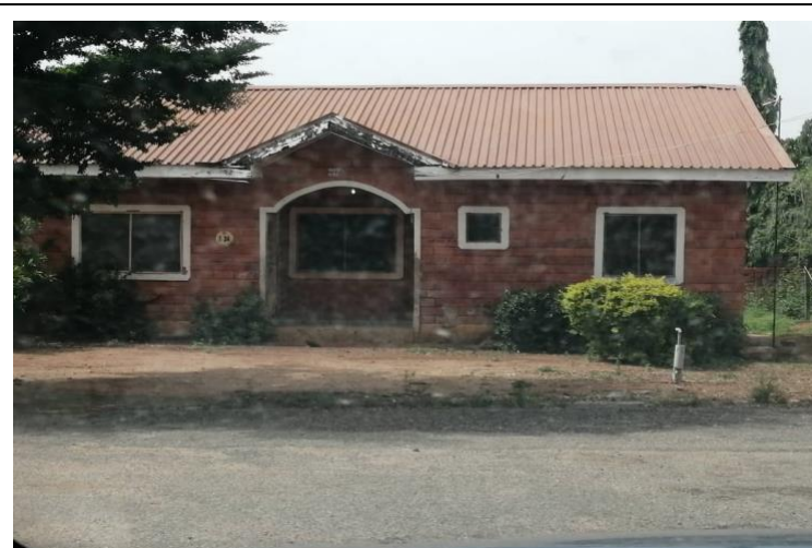
Plate 4: Another low-income scheme located on the outskirts along Suleja road. This scheme is fairly decent when compared to most of the low-income schemes with the provision of some infrastructure. However, it is poor maintained and is in a dilapidated state
